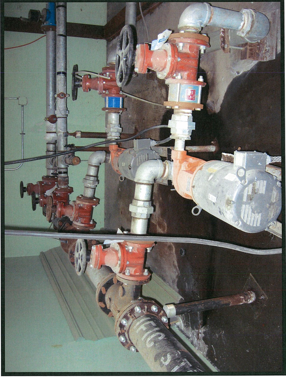
Harmony Wells Booster Pumps and System
