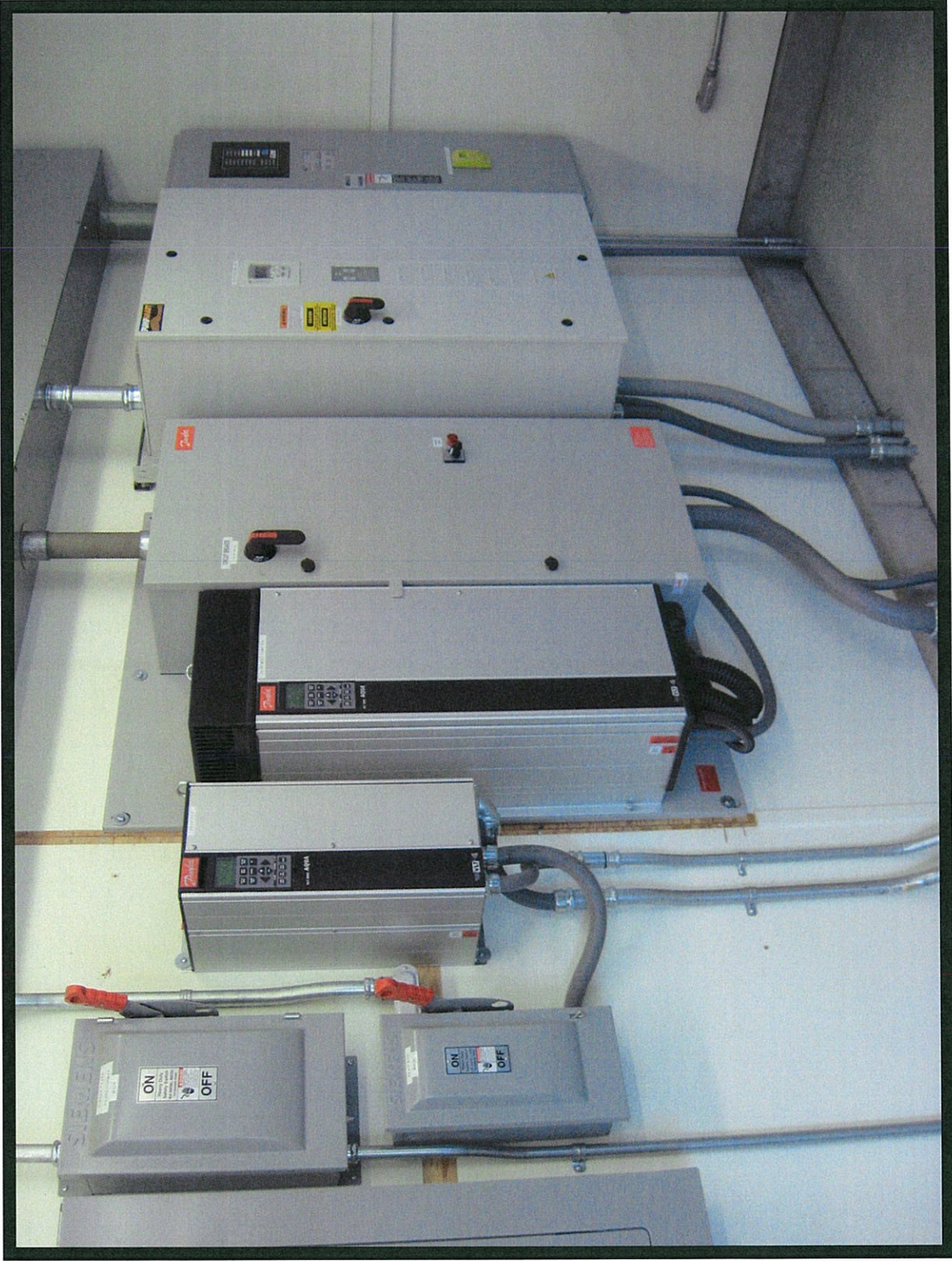
Butler Well Pump System Controlling Works
