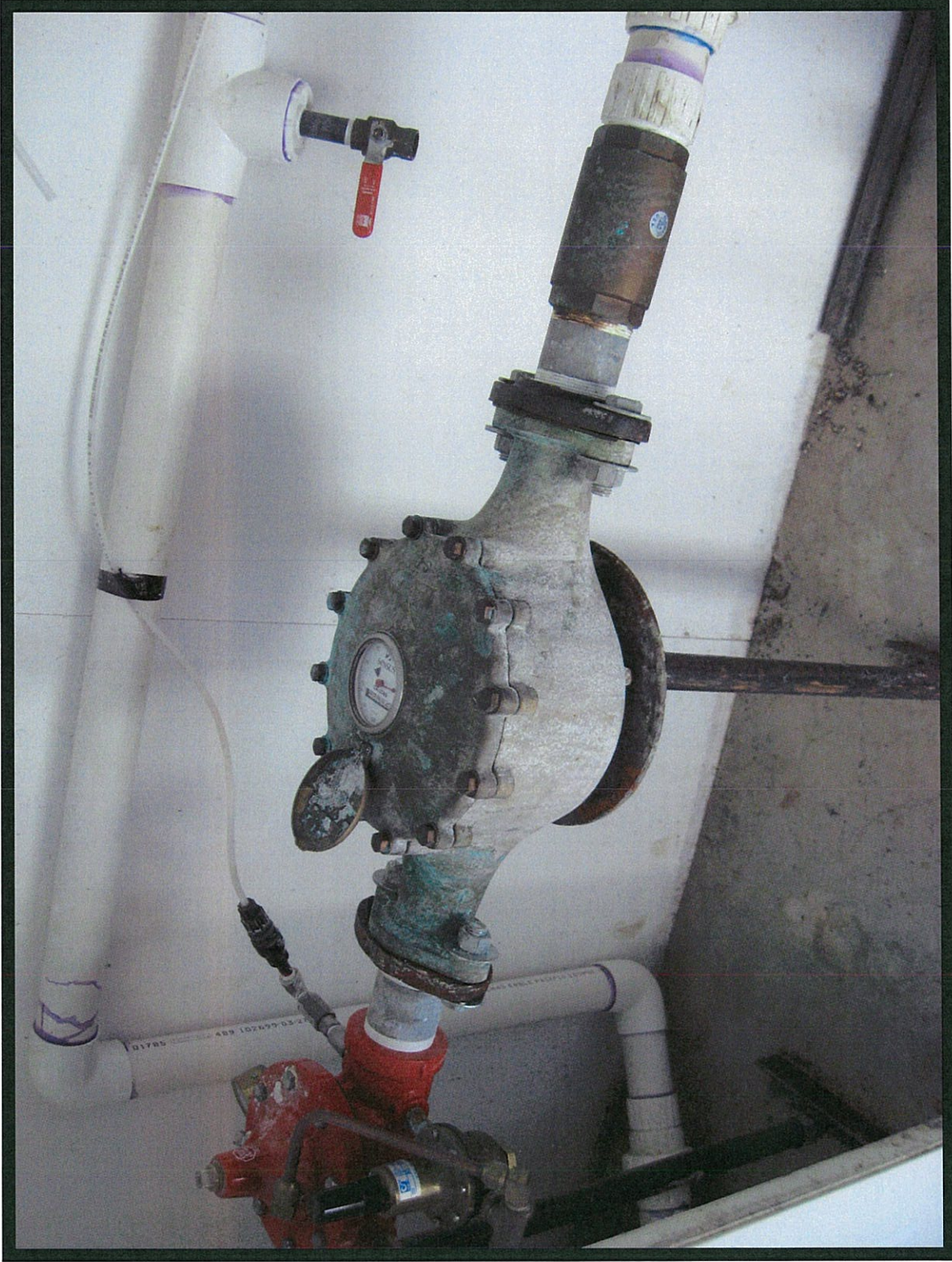
Friends Well In-line Flowmeter
