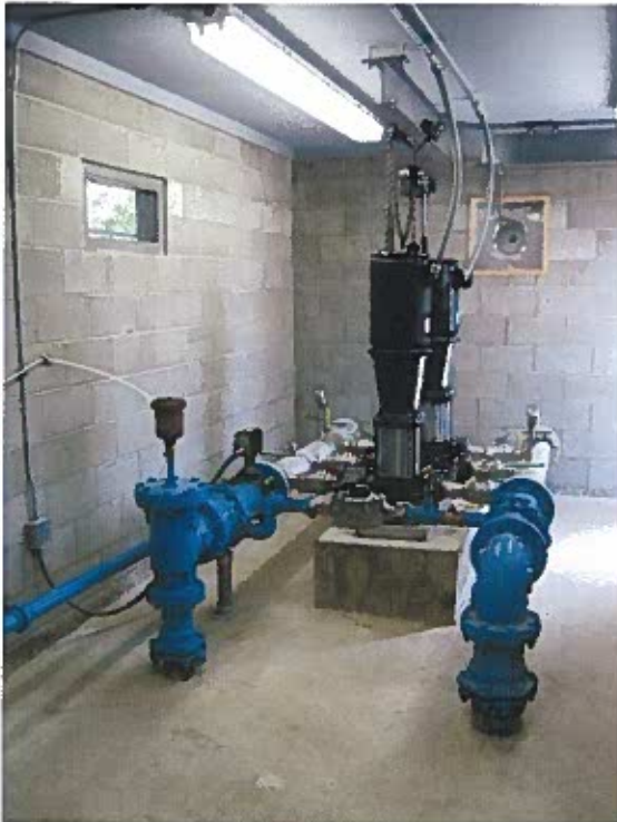
94-7383 School Well at Booster Station
