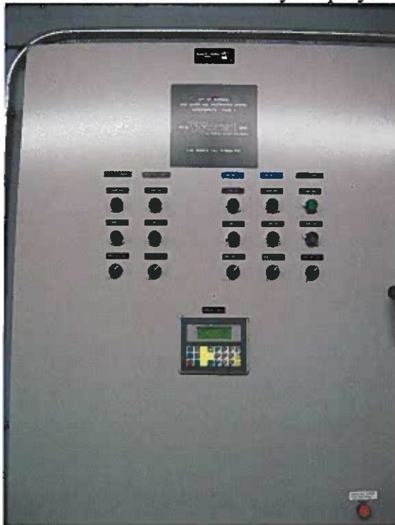
94-7383 Monitor Panel inside Booster Station
