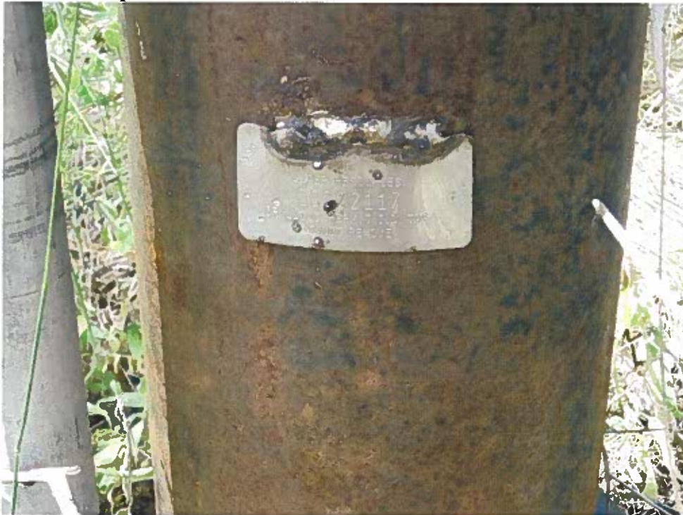
94-7383 Shop Well Two Tag Close-Up
