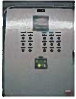
94-7383 Monitor Panel inside Booster Station.JPG
