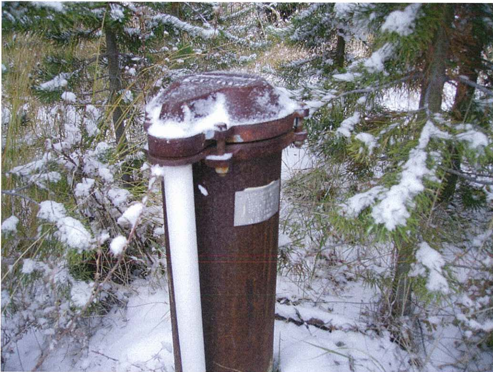
Picture 2, well head with attached metal tag, no. A0012097
