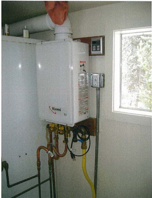
Picture 5, tank-less water heater (POU).
