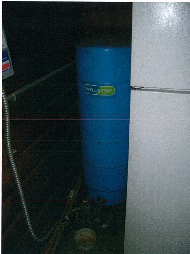
Picture 4, pressurize tank.
