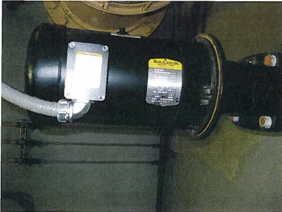
Miles AVE Baldor 3 HP Booster Pump
