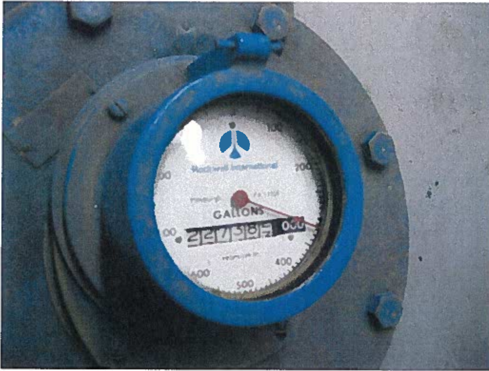
Airport Well 2 Flowmeter
