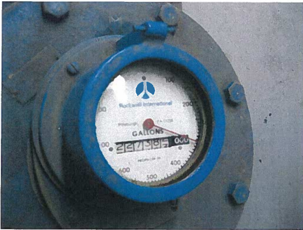
Airport Well 2 Flowmeter
