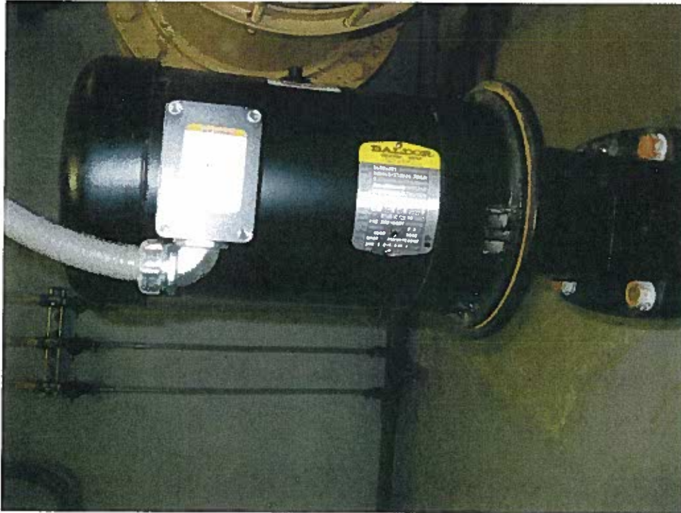
Miles AVE Baldor 3 HP Booster Pump
