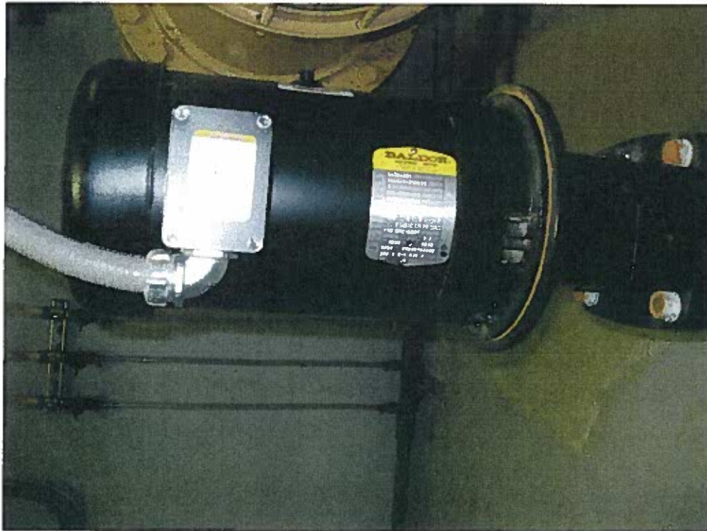
Miles AVE Baldor 3 HP Booster Pump
