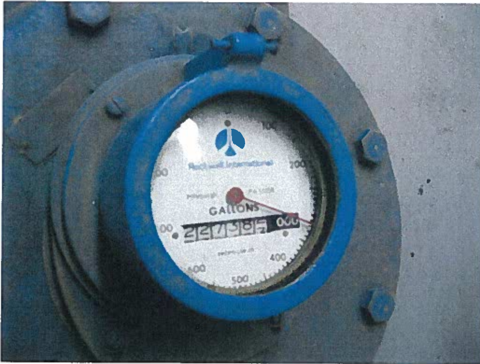
Airport Well 2 Flowmeter
