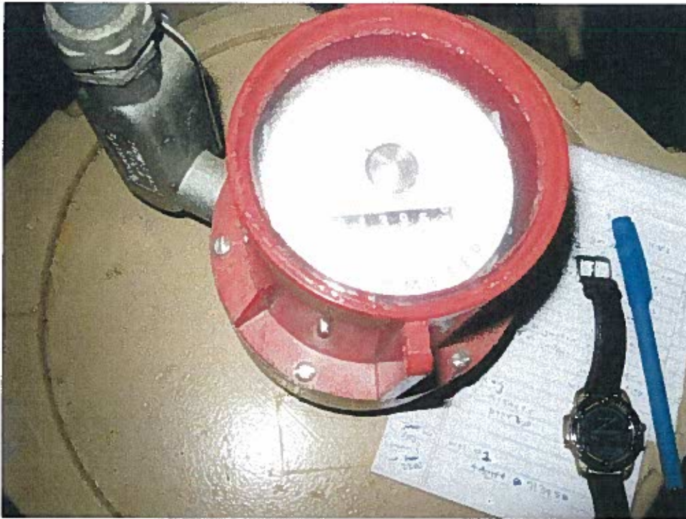
Miles Control BLDG Flowmeter Wells 1-3
