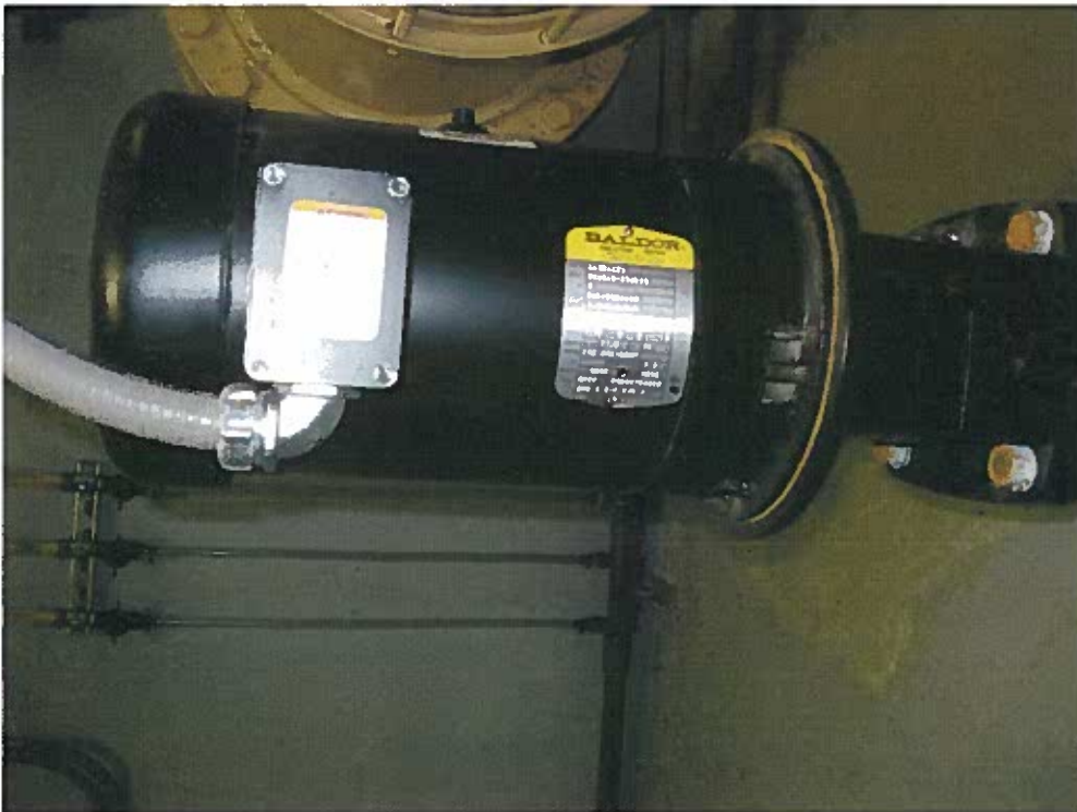
Miles AVE Baldor 3 HP Booster Pump
