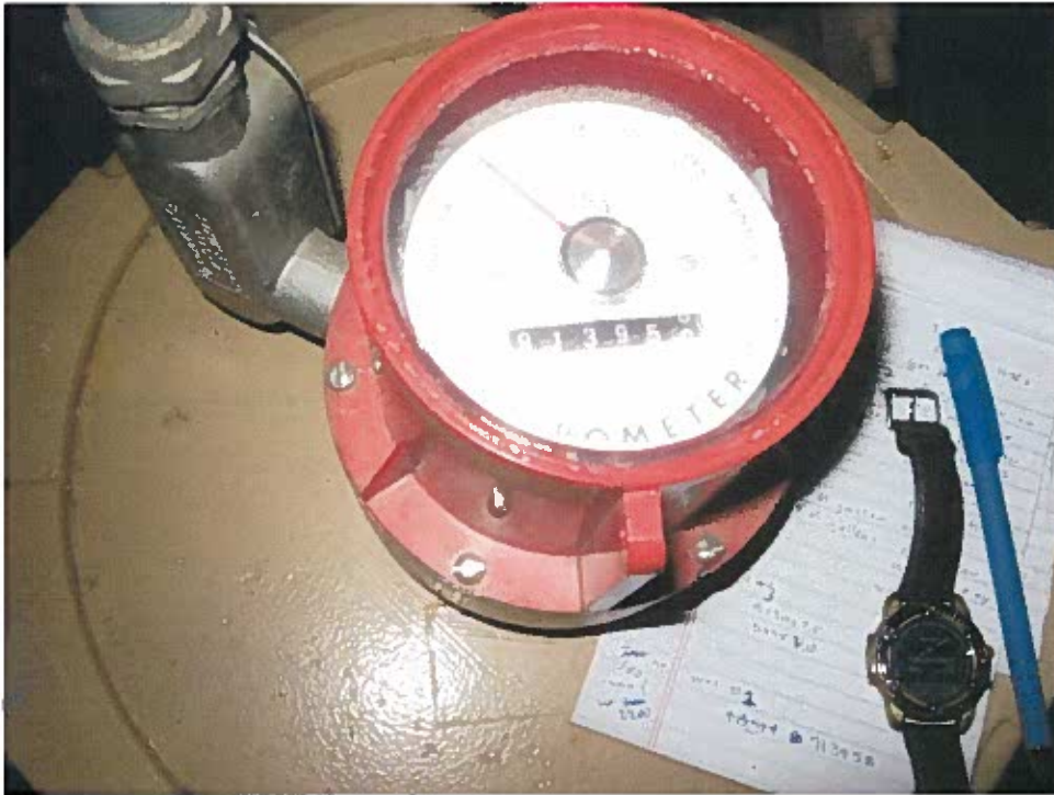
Miles Control BLDG Flowmeter Wells 1-3
