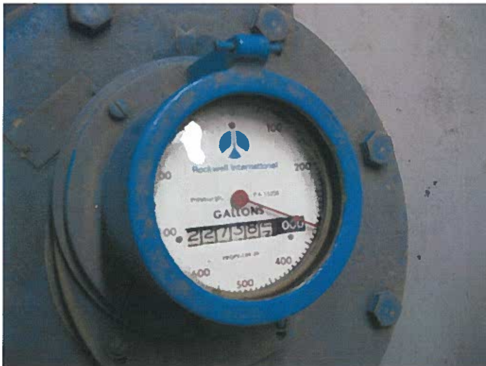
Airport Well 2 Flowmeter
