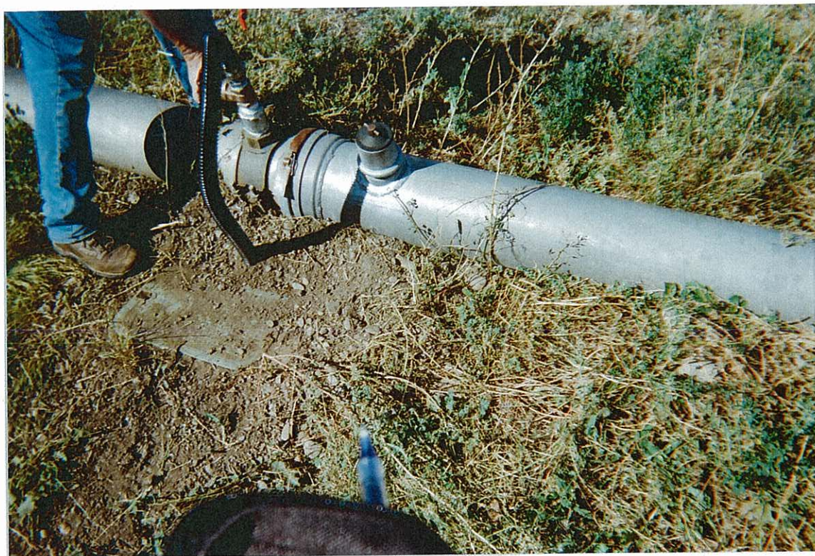
Irrigation pipe with line to pump
