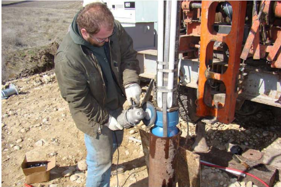
Figure 18. Pump and Motor Assembly used in the SVR #7 Test
