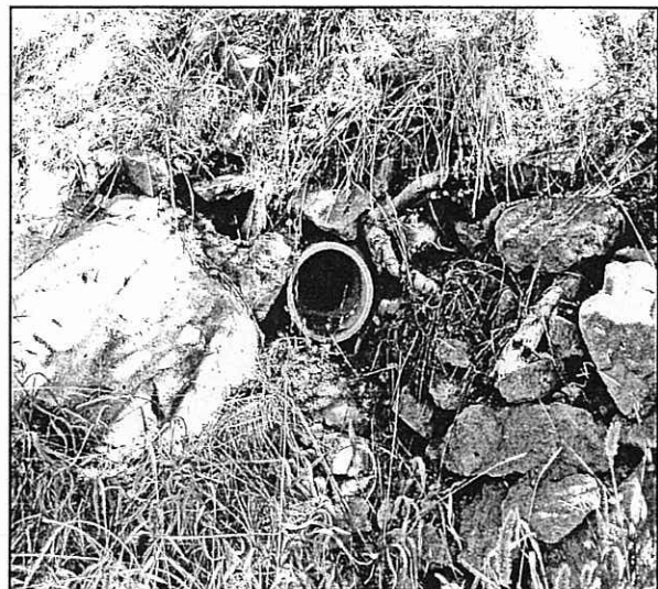
Fig. 19 – storage tank drain
