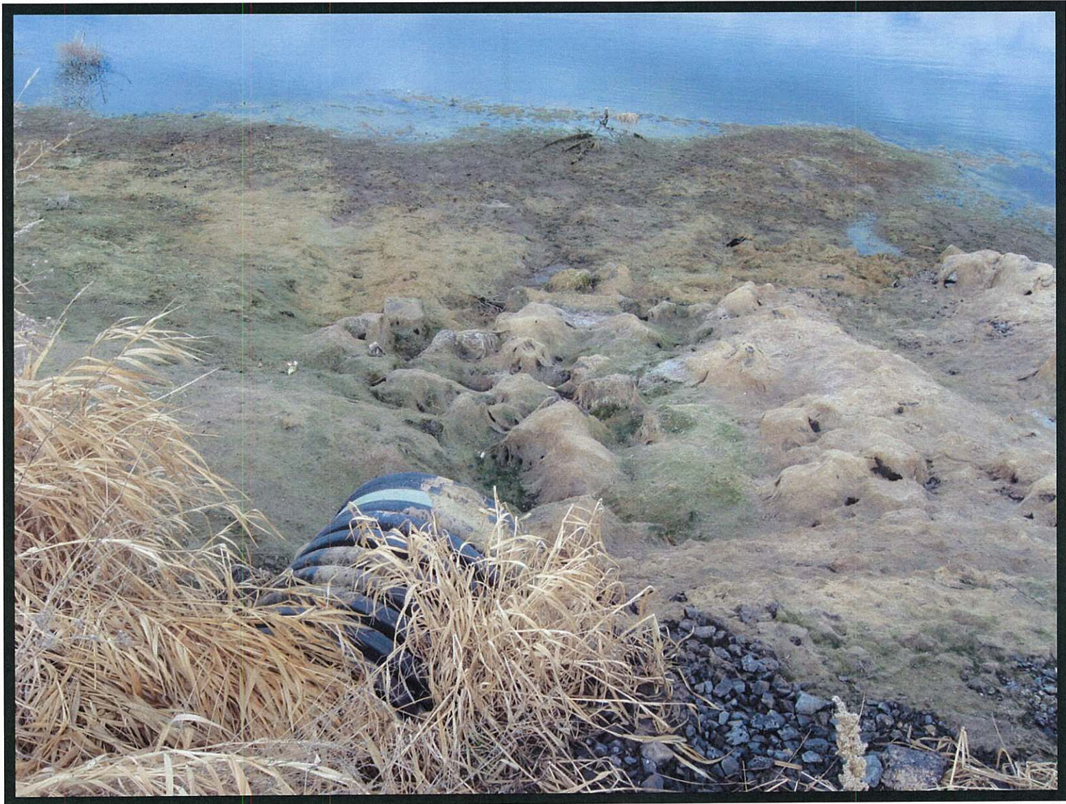
Discharge Pipe for Surface Water Located on East Side of Pond (just west of well)
