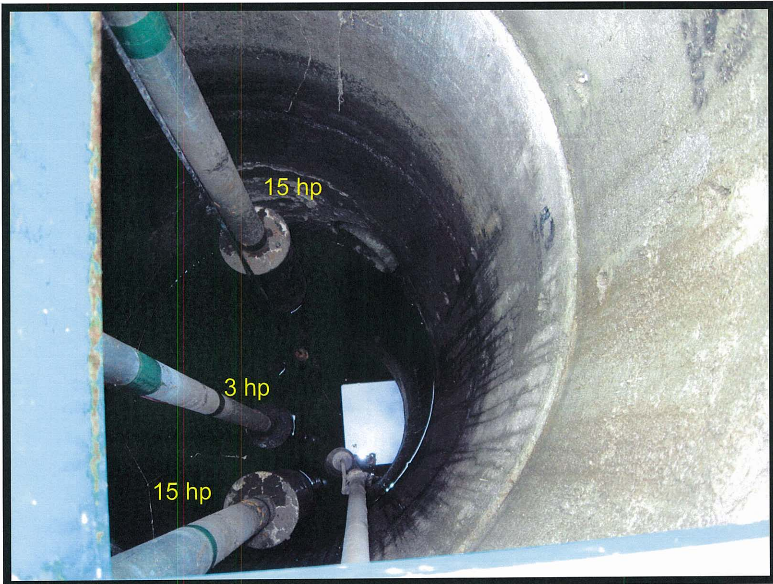
Wet Well & Three Submersible Pumps
