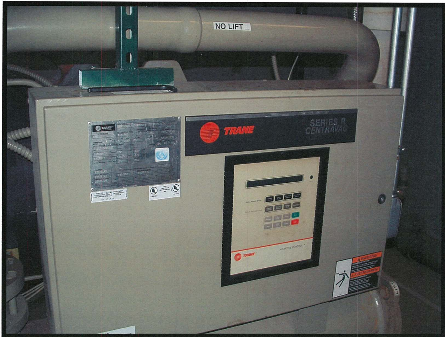
Trane 240 Ton Chiller/Condenser Cooling System
