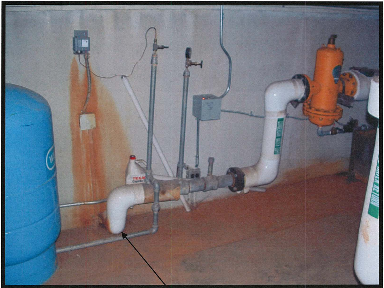
Entrance Pipe from Well to Cooling System
