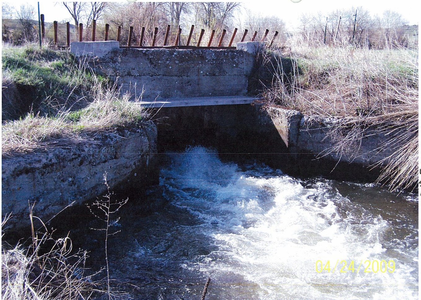
Head Gate w/ Submerge Orifice Weir
