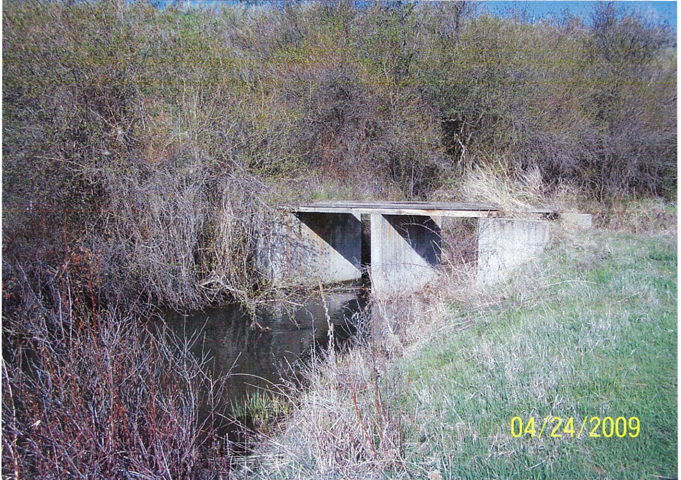
Flood Control Device
