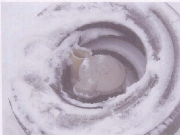
East Well @ Barn 1
