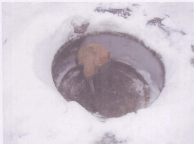
West Well @ Barn 1
