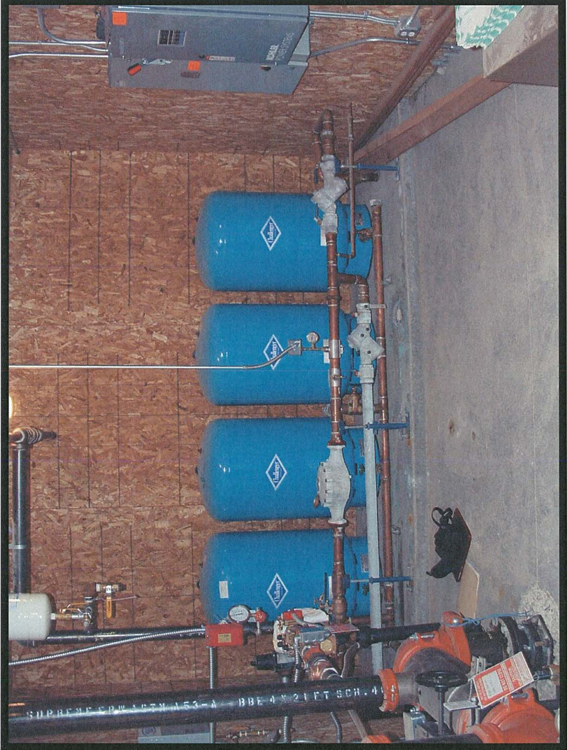
Domestic Storage Tanks and Pipe System
