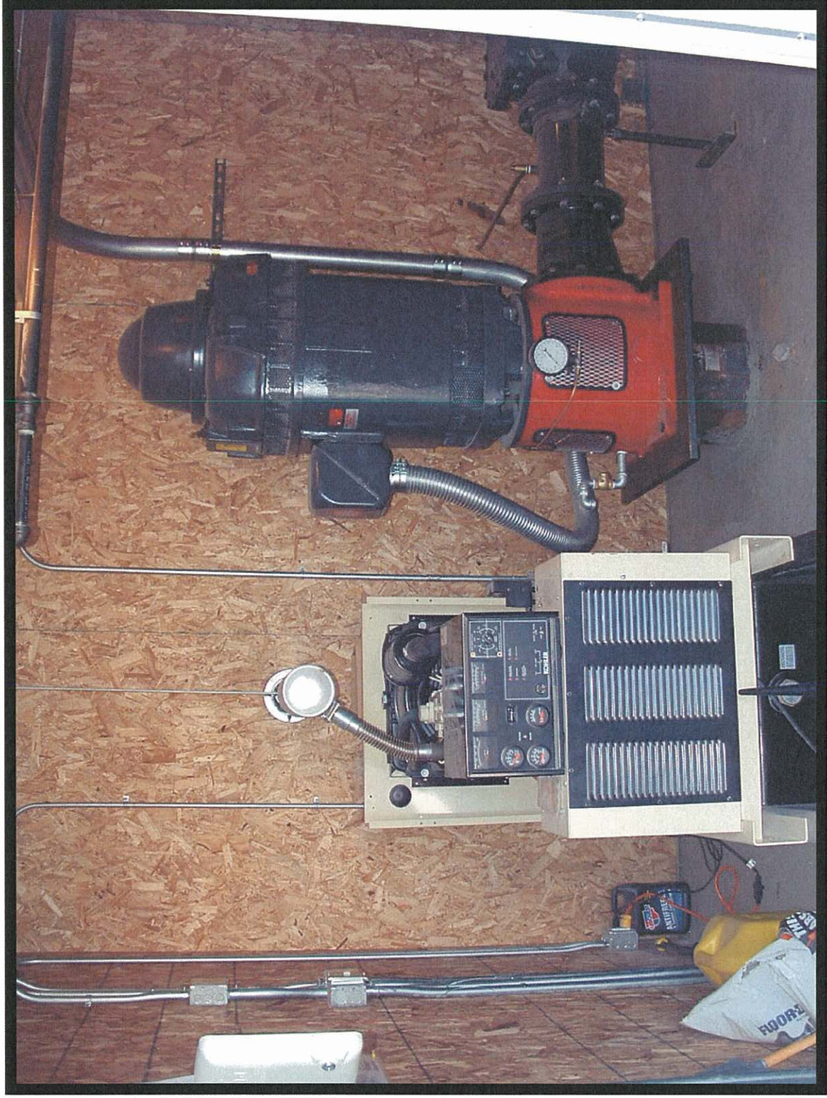
Well, Pump and Back-Up Generator
