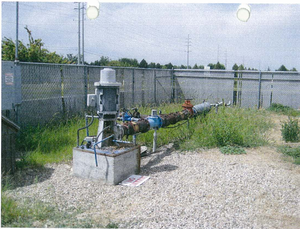
Photo 3 taken facing west--pump system that draws water from pond and distributes the water for irrigation
