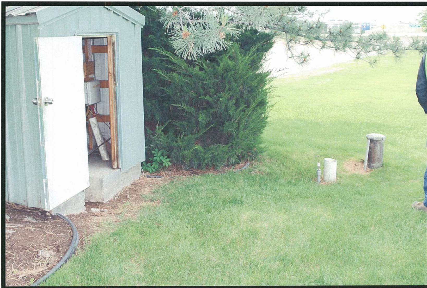
8-inch Well and Well House
