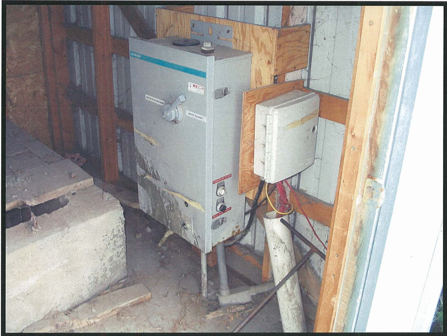
Pump Controlling Works
