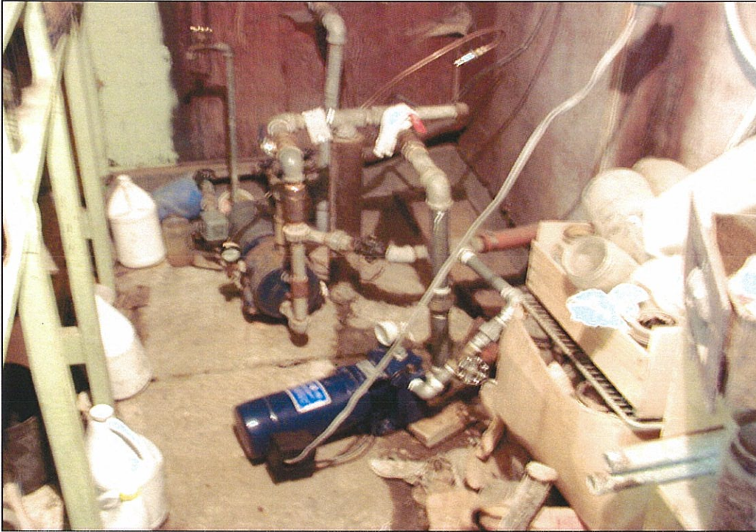
Well head looking West in building. Dairy / House Well, 5/13/03, 13:37 hrs, photo by Chris Duncan - Holladay Engineering Company. Photo 1
