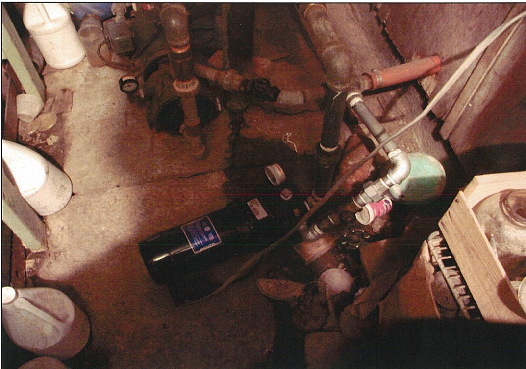
Well head looking West in building. Dairy / House Well, 5/13/03, 13:37 hrs, photo by Chris Duncan - Holladay Engineering Company. Photo 2
