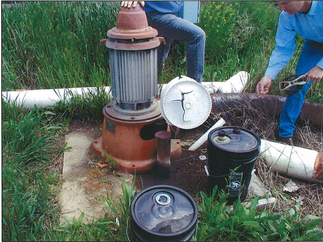
Looking East at well head. Big irrigation well, 5/13/03, 14:15 hrs, photo by Chris Duncan - Holladay Engineering Company. Photo 11
