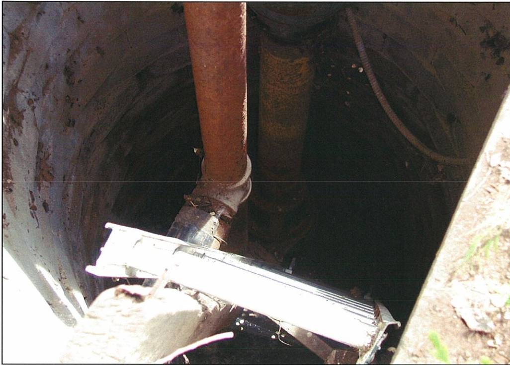
Well head. Small irrigation well, 5/13/03, 13:56 hrs, photo by Chris Duncan - Holladay Engineering Company. Photo 5
