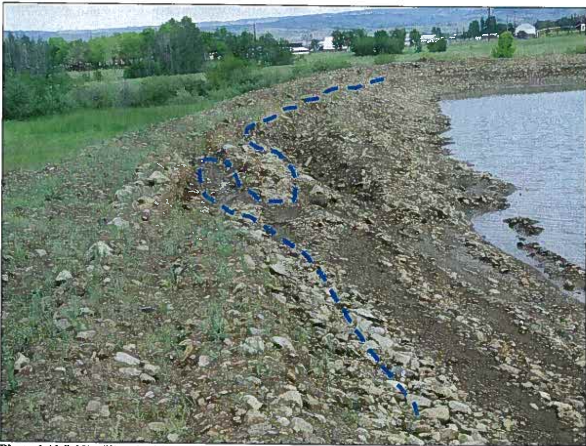
Photo 1 (6-5-09) - View looking north along the western, centerline axis of the existing embankment dam. The pool level is approximately 4 feet lower than first observed yesterday when it was within just a few inches from overtopping the dam, as indicated by dashed line. At its narrowest dimension, the dam crest is only about 6 feet wide. Construction materials were obtained from the pool area and pushed up to create the perimeter embankment. The dam was built without IDWR dam safety approval; neither was it designed by a licensed professional engineer.
