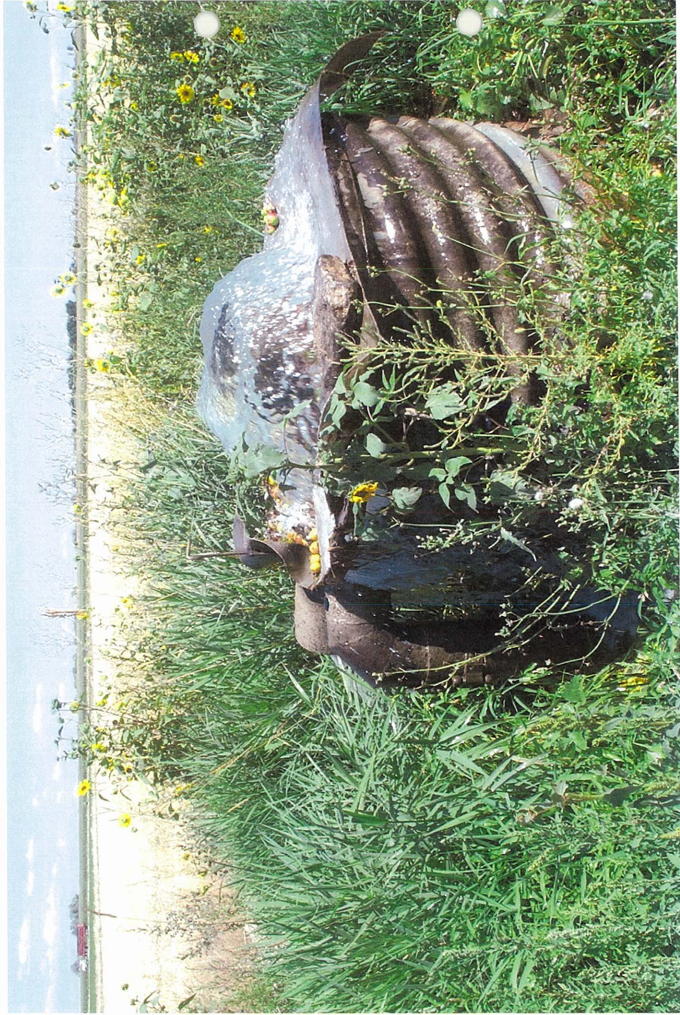
47-7861 Naves Water cleaner In Ditch Looking East 8-17-09 By J Stanton
