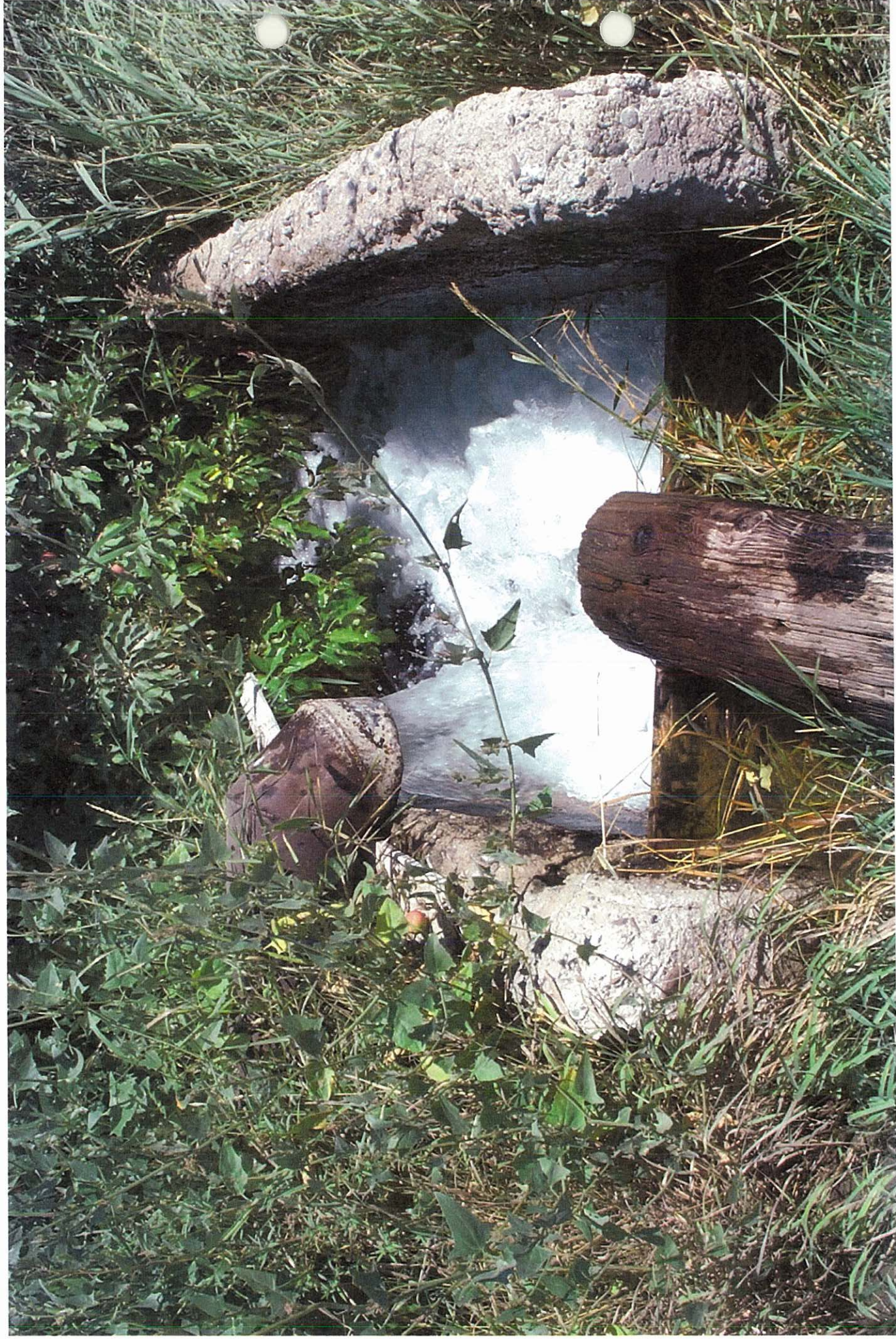
47-7861 Nunes Well Discharge Into Ditch (Looking East) 8-17-09 By J Stanton
