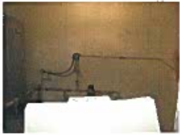
inside pump house.JPG
