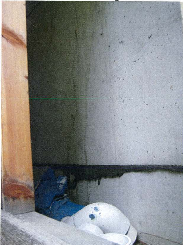
Photo 3: The cement storage tank
