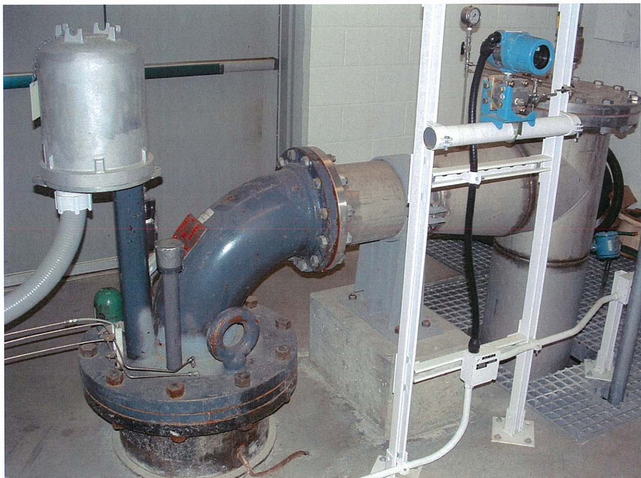
Micron Well No. 5 (injection) wellhead (on left) for ground-water recharge at Building 31.
