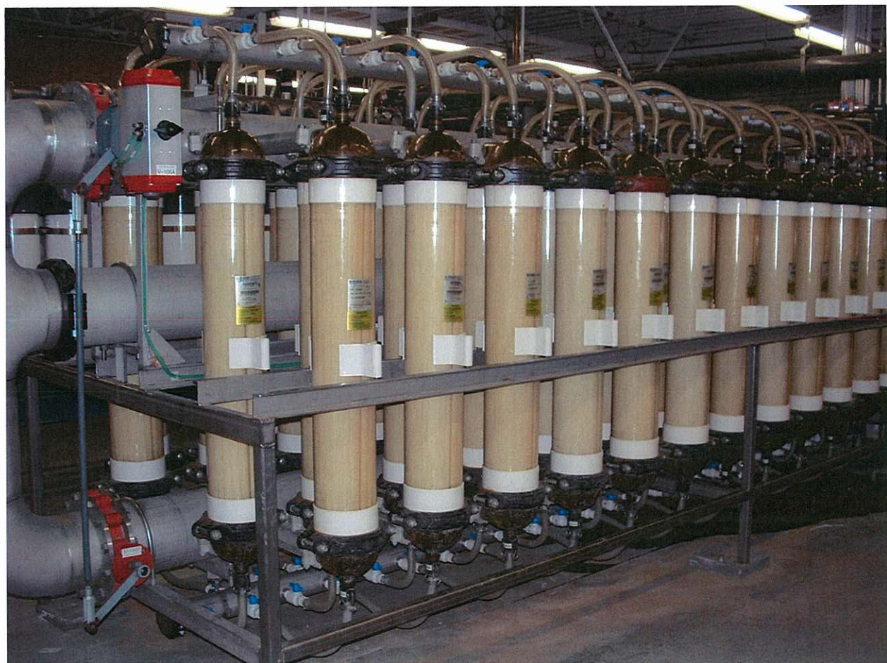
Ultrafiltration skid No. 100 at Building 31.
