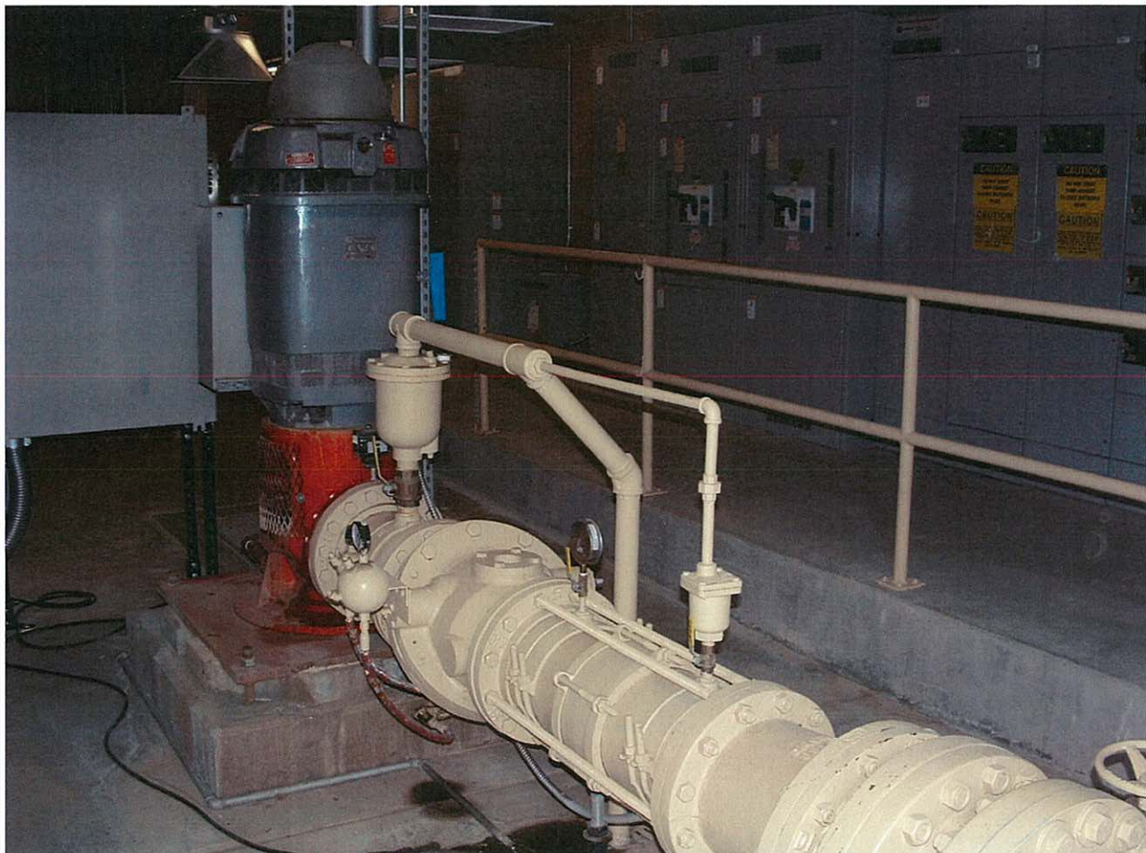
River water pump 1, 200-hp variable speed motor.
