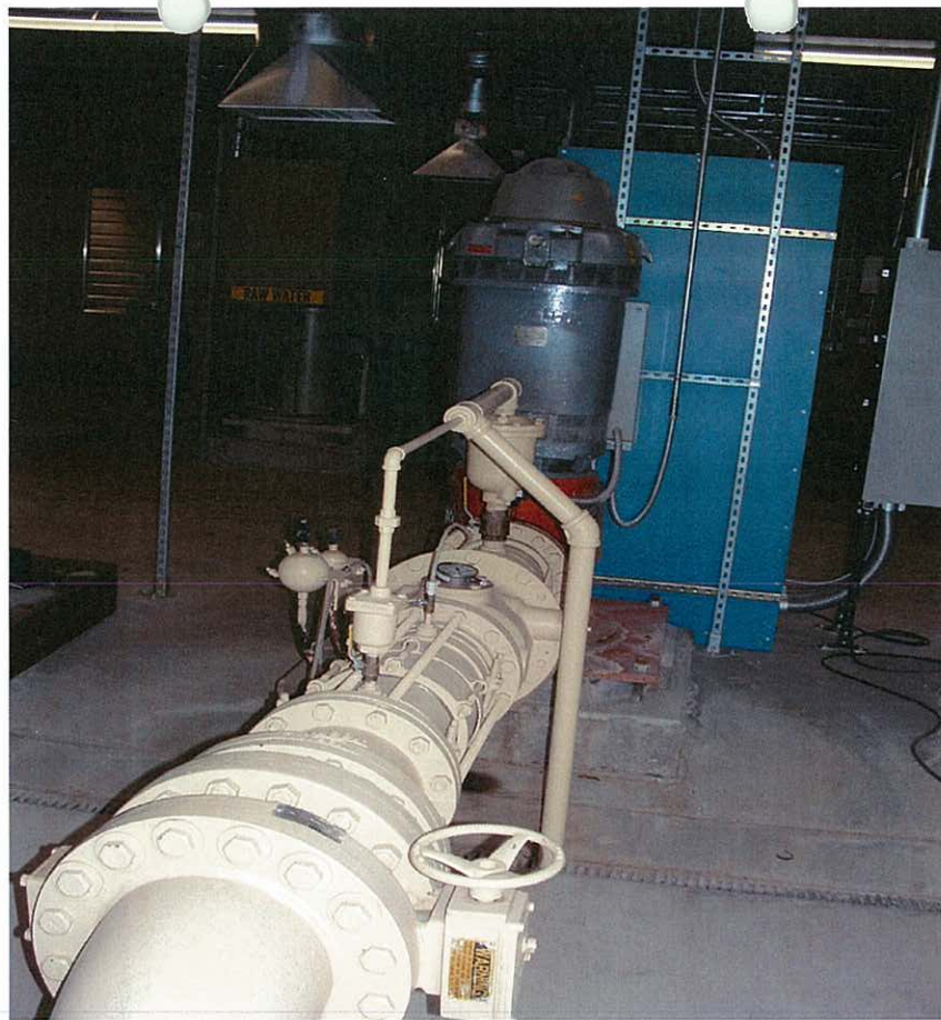
River water pump 2, 200-hp variable speed motor.
