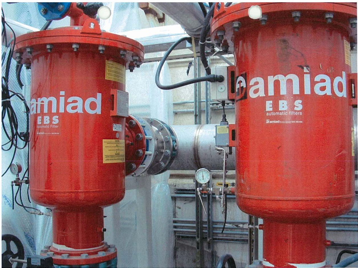
Filters at entrance to Micron plant at Building 22, upstream from heat exchangers.
