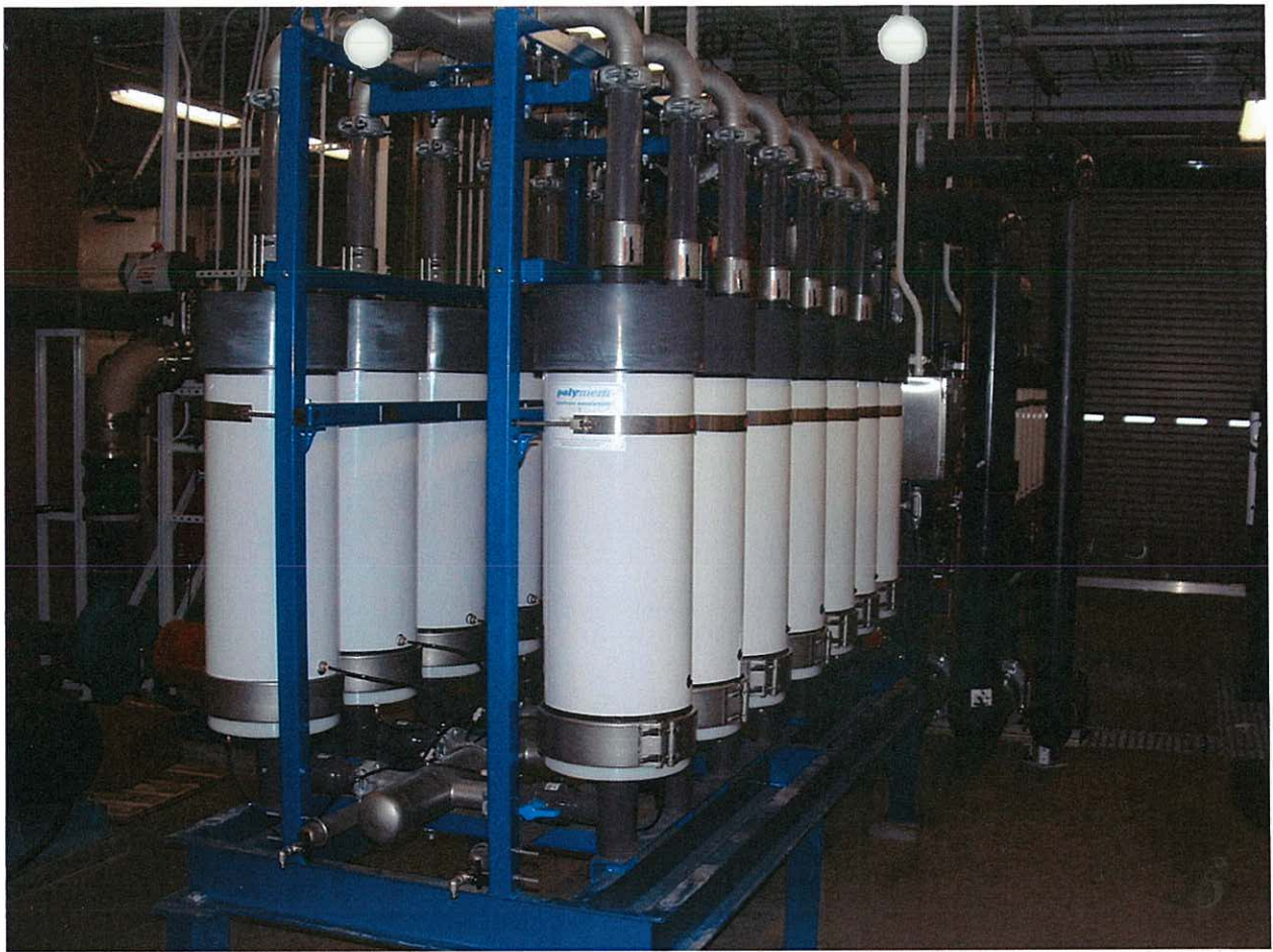
Ultrafiltration skid No. 200 at Building 31.
