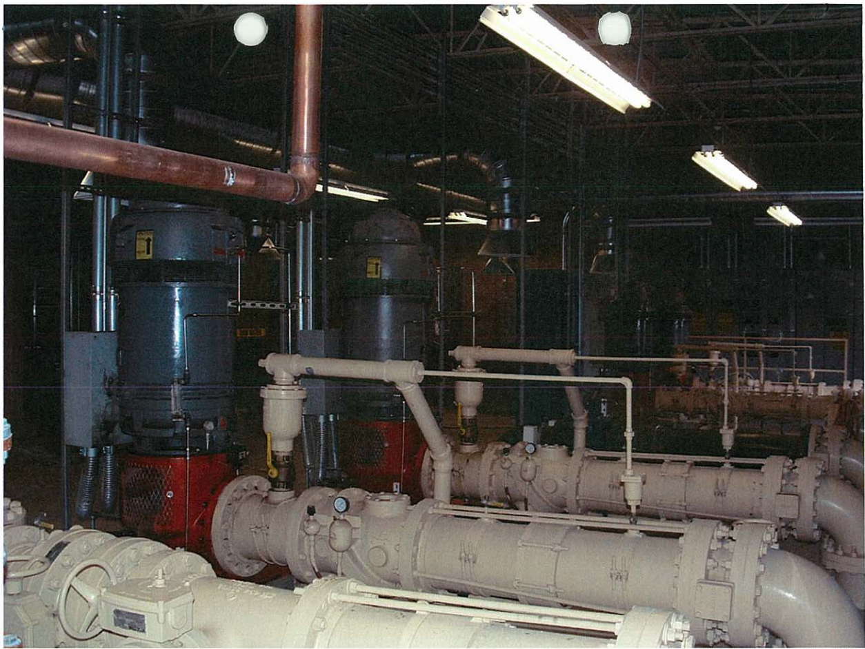
View of four pumps. River water pumps 5 and 6 in foreground. Pumps 1 and 2 in background.
