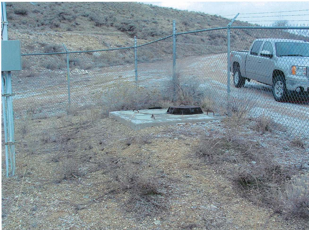
Flow meter vault on west side of Boise River pump station.
