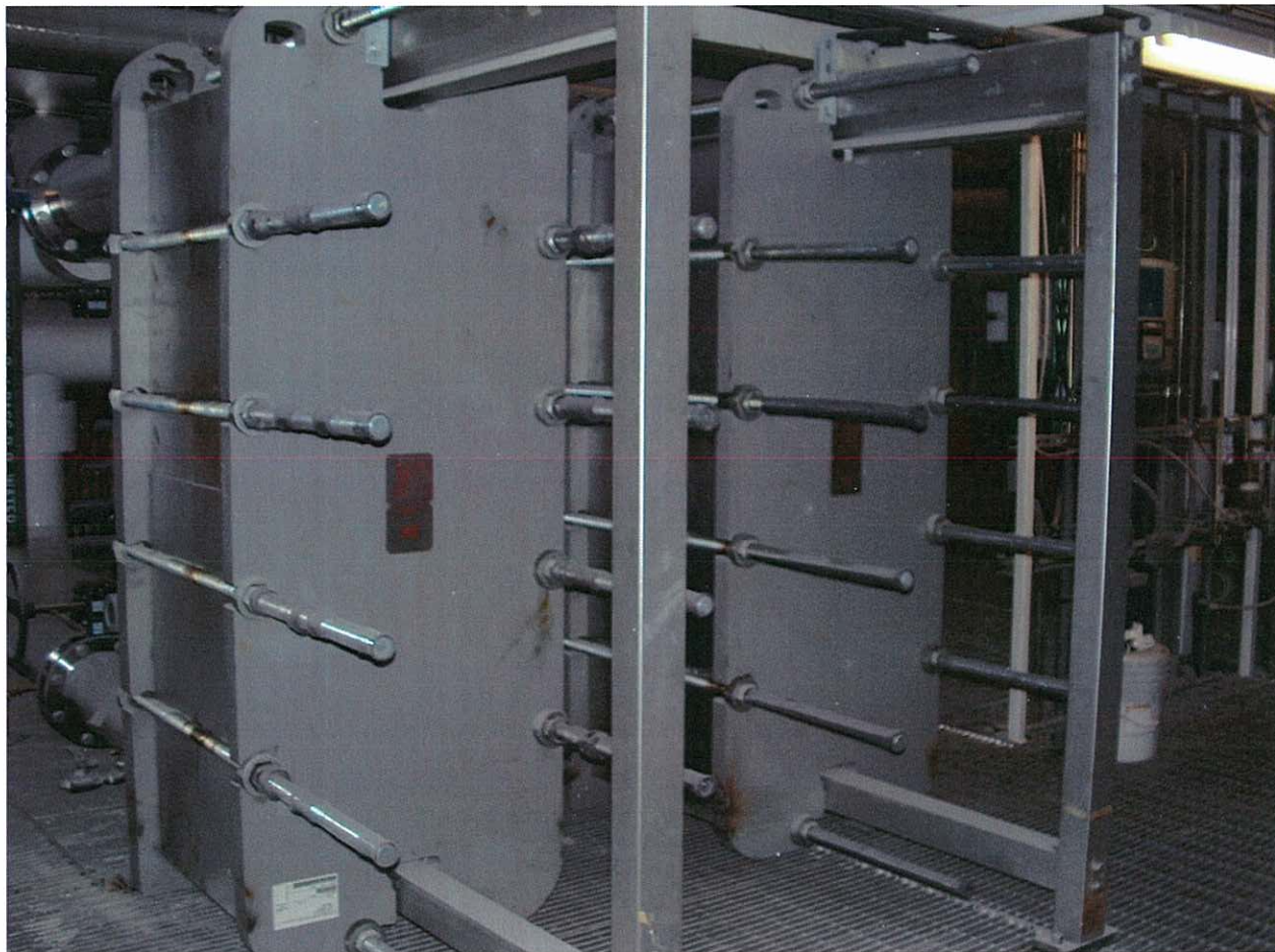
Heat exchangers in Building 22. All water diverted to plant goes through the heat exchangers.
