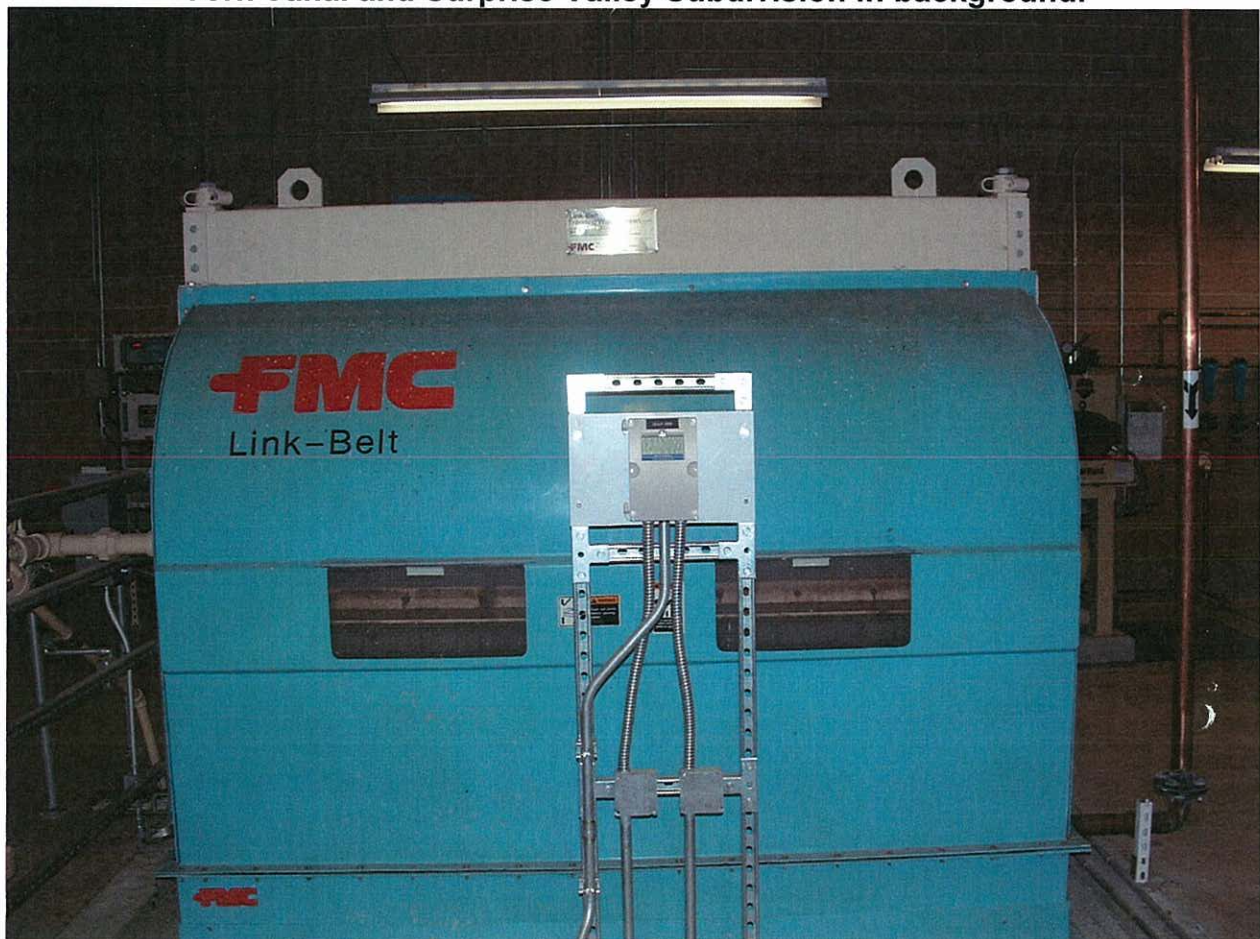
Traveling screen enclosure within pump station.
