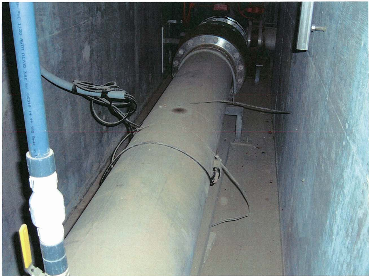
Well 5 ultrasonic flow meter at Building 31.
