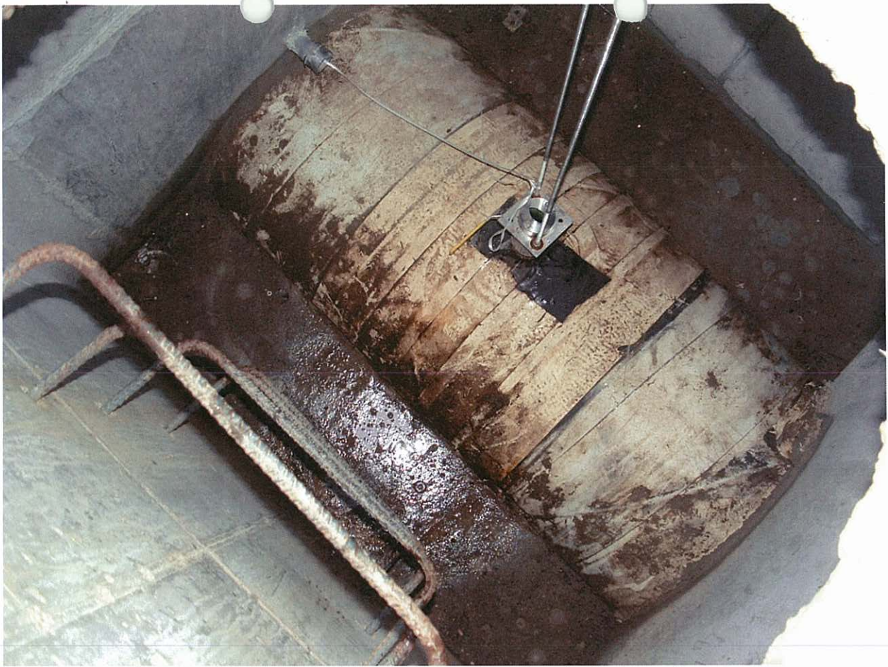
Flow meter tap on 30-inch diameter pipe in flow meter vault.
