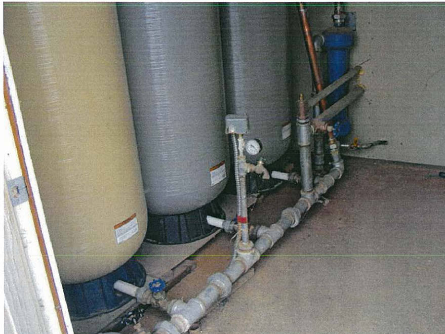
Pump House System & Well Located in the SESE S9 T2S R2W AKA Lot 6, Block 2
