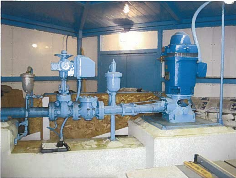
95-8057 Well BLDG Interior
