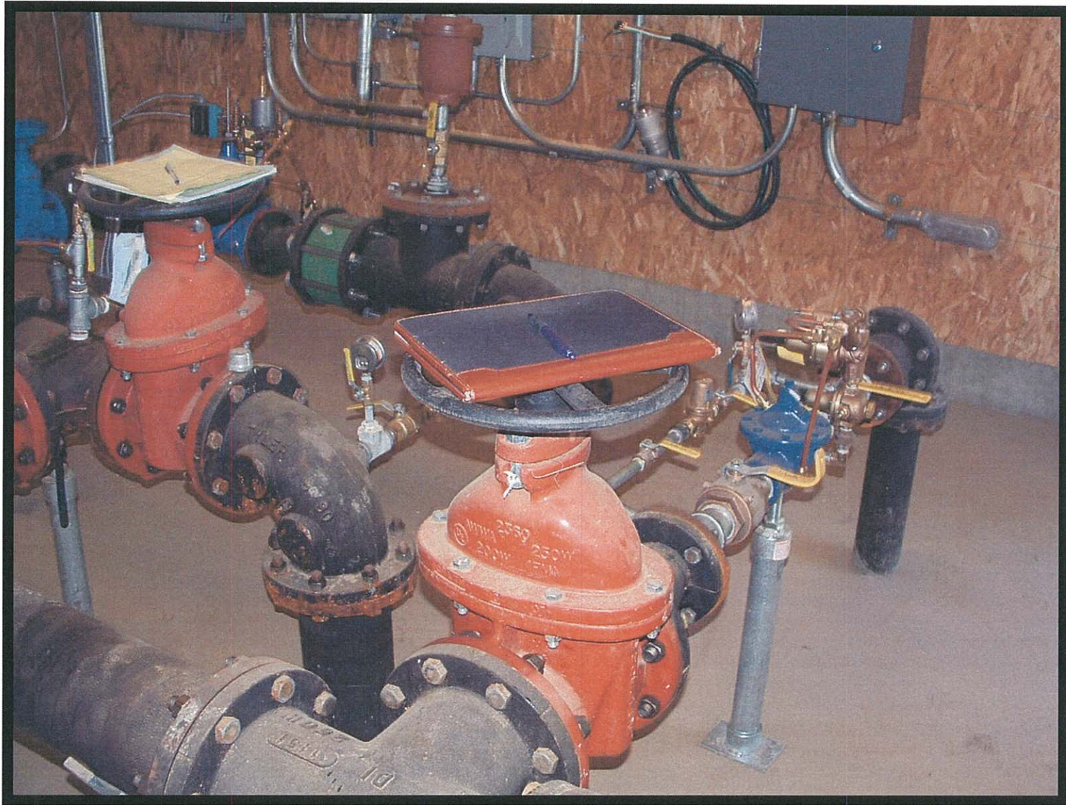
Controlling Works in Well House
