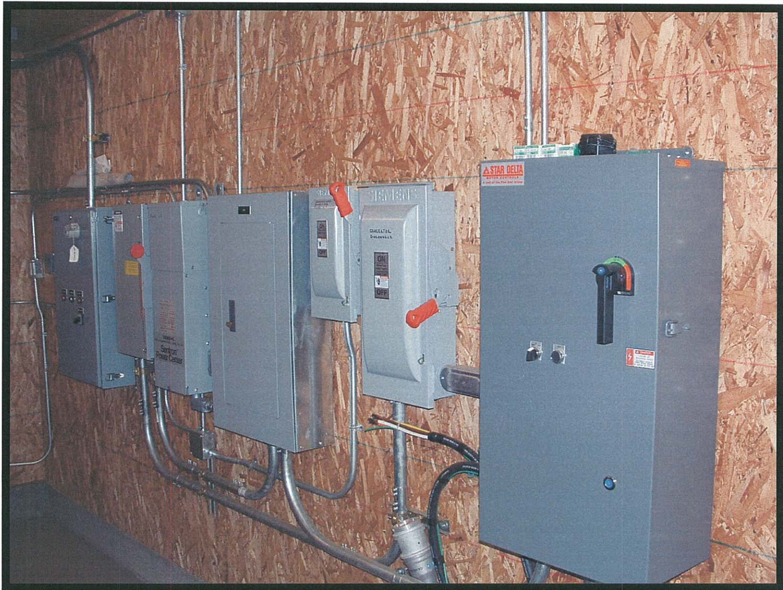
System Control Panels in Well House
