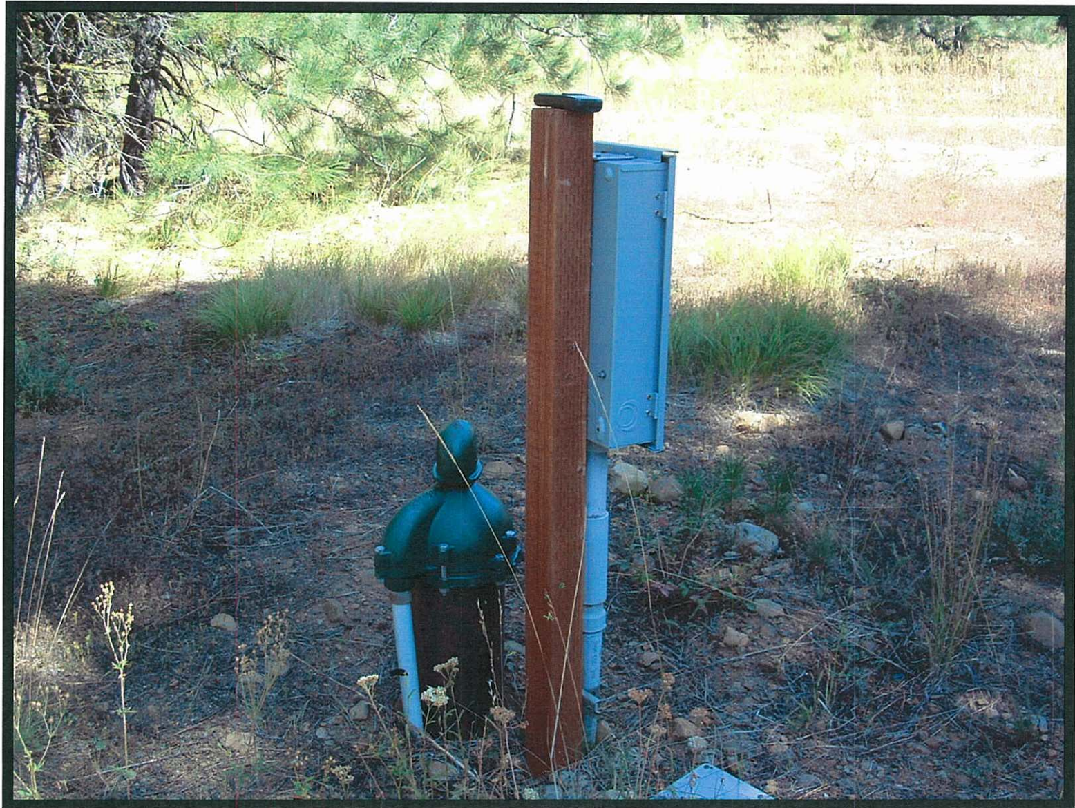
North Well and Pump
