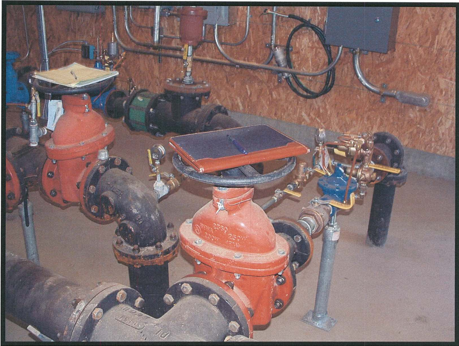
Controlling Works in Well House
