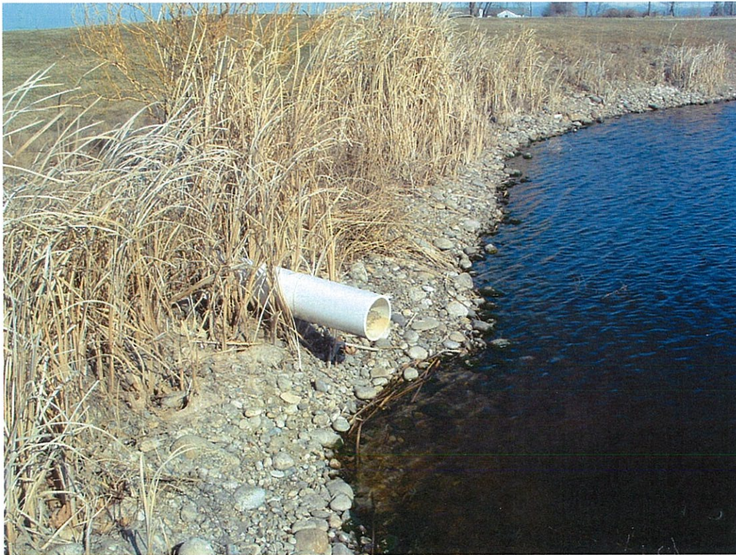
8-inch pipe inlet to pond from well
