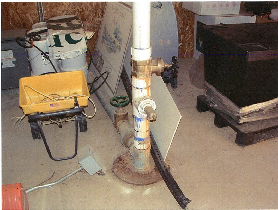
View of well head. Horizontal pipe is discharge to pond. Vertical pipe to truck fill.
