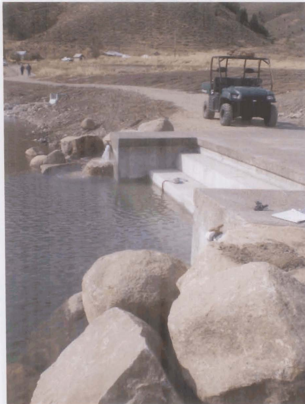
Valves on either side of terrace allow introduction of hot water directly at the step area.
