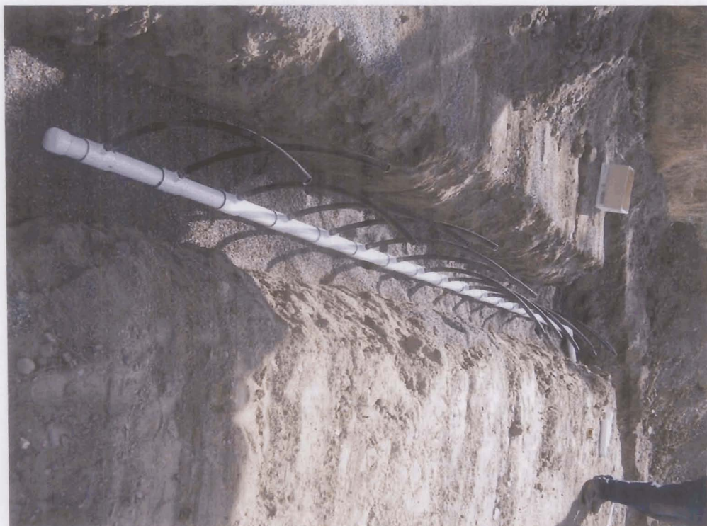
Example of snowmelting zone header (photo date 9/15/09)
