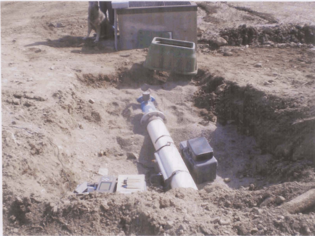
Flow meter on inlet pipeline to collection box Portable ultrasonic meter installed for comparison
