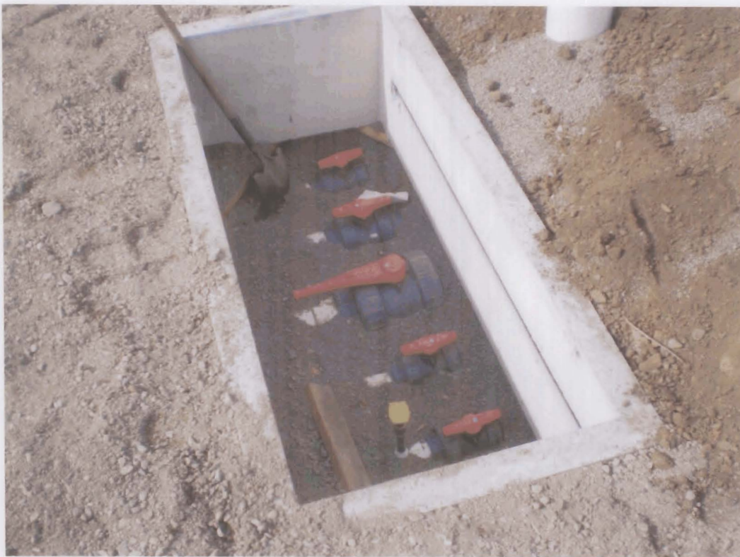
Main manifold. 4" valves to snowmelting system; 6" valve in mainline to pond.
