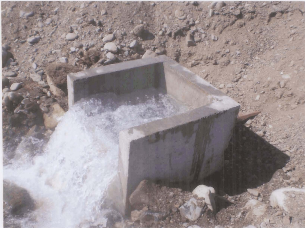
Discharge to pond / spa
