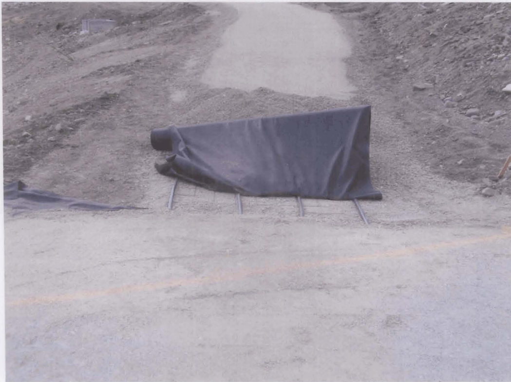
Example of snowmelting radiator placement (photo date 9/15/09)
