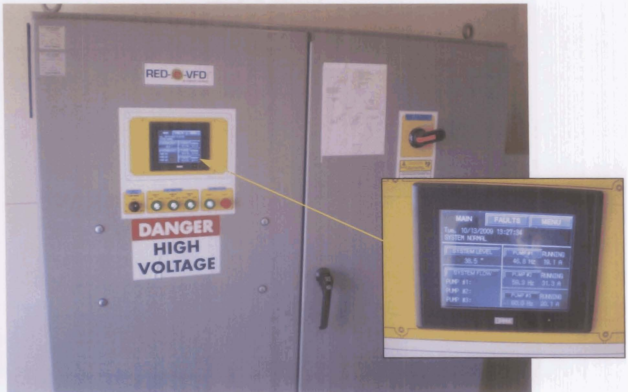
Variable-frequency controller and 3-phase converter
