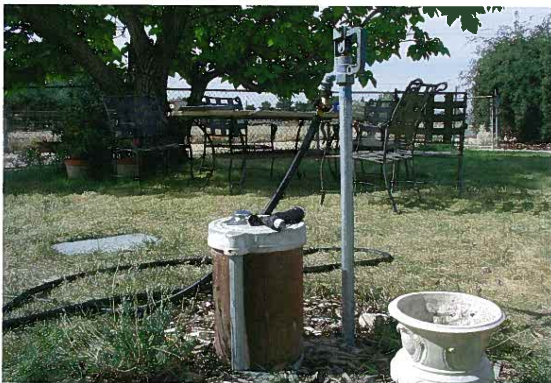
Well with 5 hp submersible pump. Located behind (east of) house. 8" casing.
