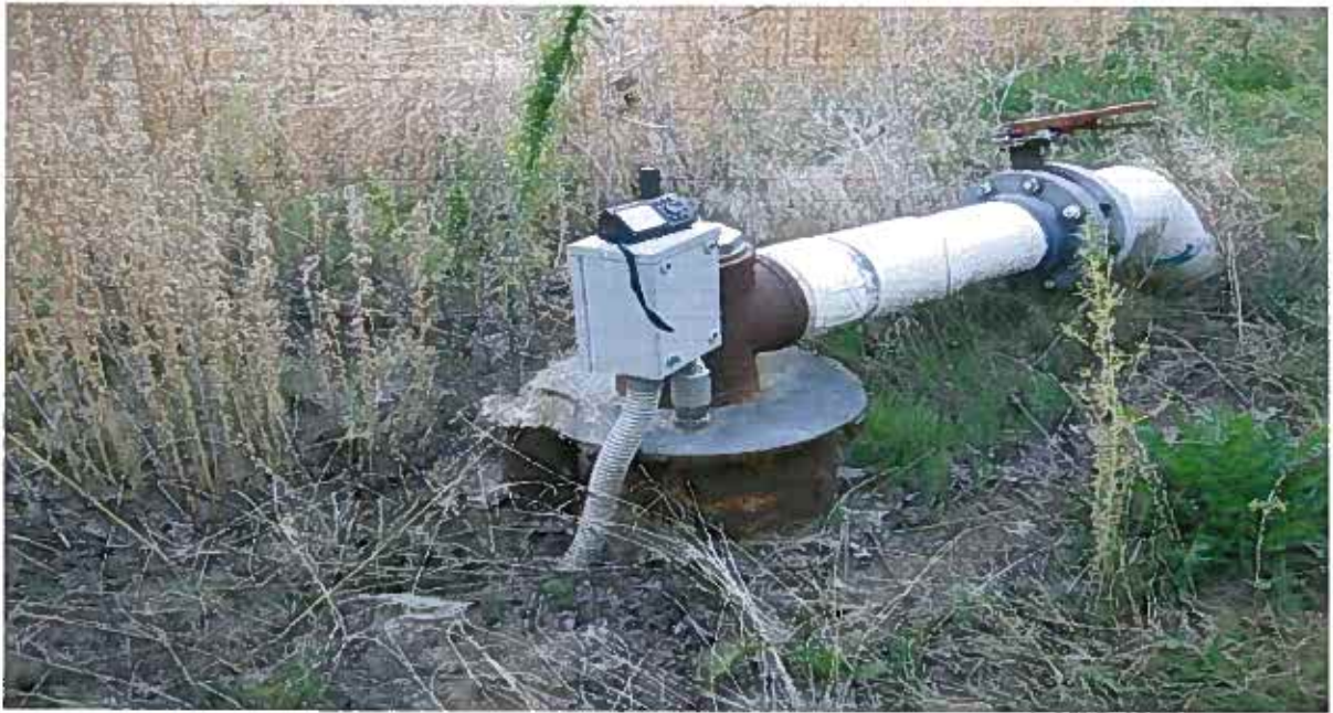
Point of diversion – 12" diameter well located by shop. Section 23 SWNE
