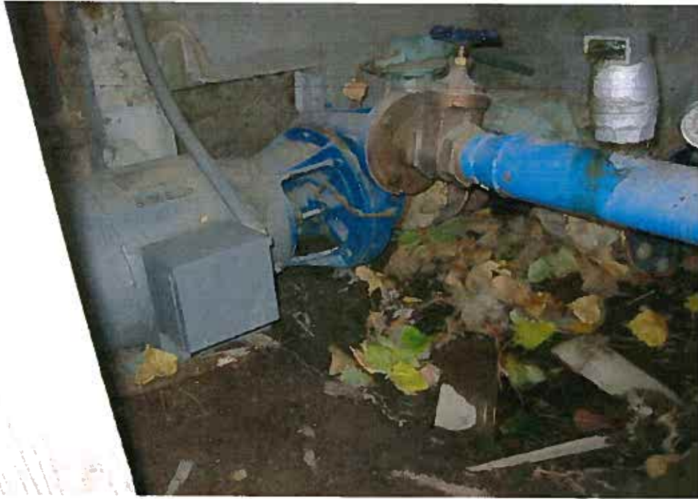
Diversion/delivery system - Interior of pump station that is located north of shop and irrigation box. Purpose is to pressurize the line from the well. 10 hp GE pump.
