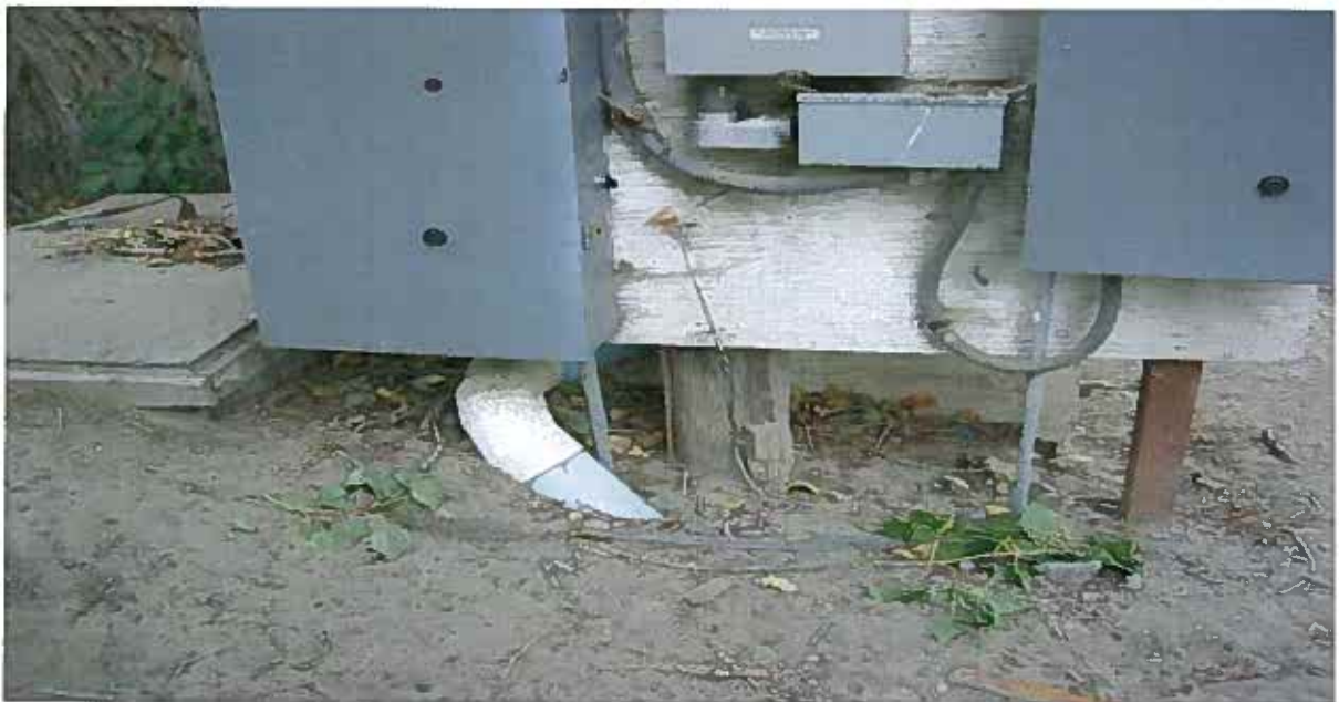
6" pipe from well into irrigation box located south of shop and well.
