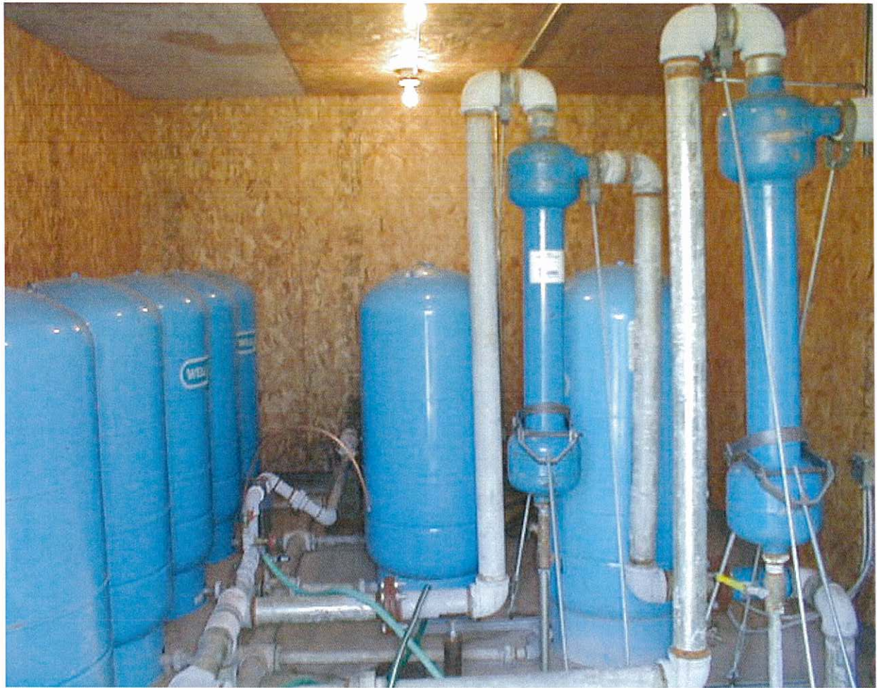
Picture No. 13; Visible lines, sand filters, pressure tanks, and sample tap.
