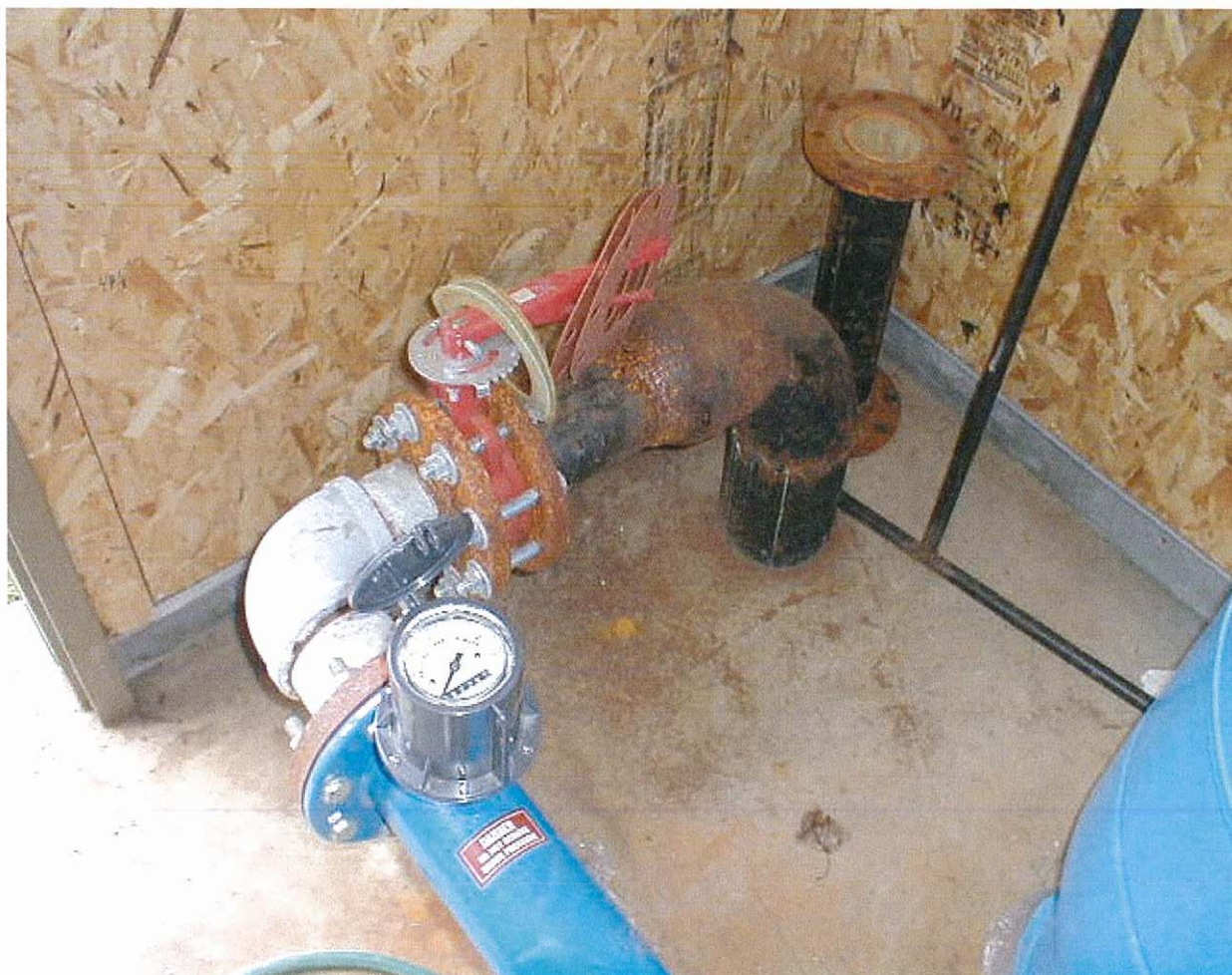
Picture No. 7; Line into tanks from the wells, isolation valve, and flow meter.
