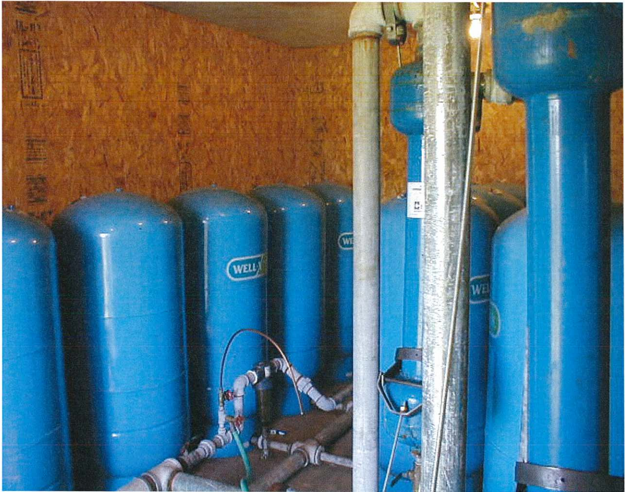
Picture No. 9; Pressure tanks 7 through 10, visible lines, and sand filters.
