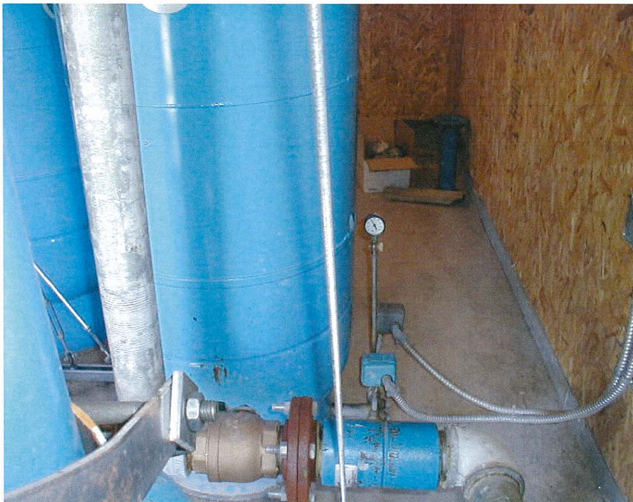
Picture No. 12; Pressure switch and pressure gauge.
