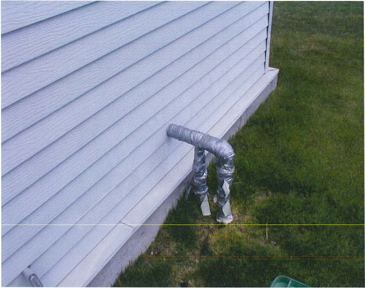
Picture No. 5; Sprinkler exit line from the shed to the system.
