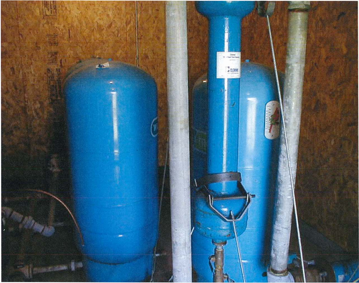
Picture No. 10; Sand filter.
