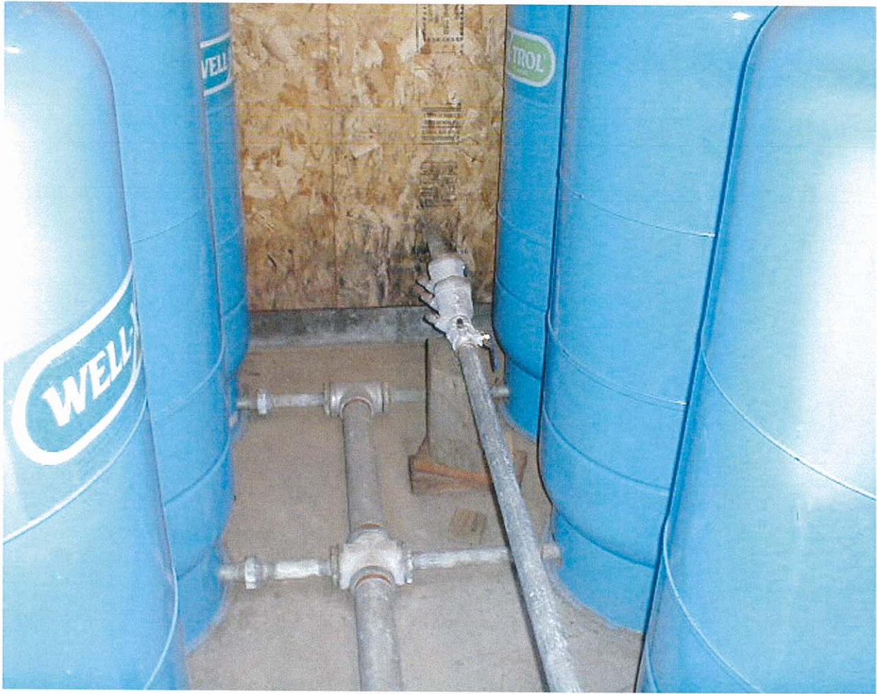
Picture No. 11; Lines from tanks and double check valve for irrigation system.
