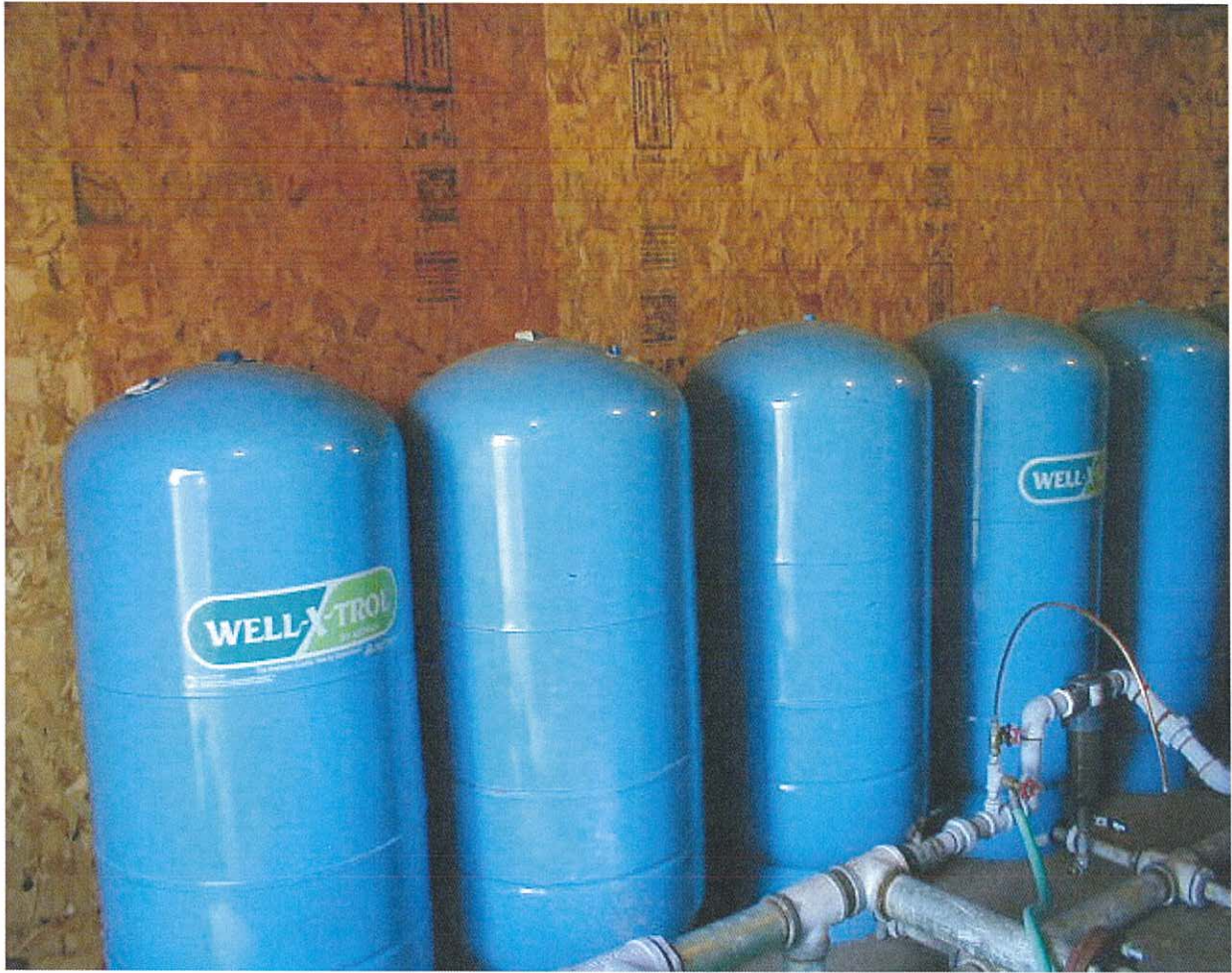
Picture No. 8; Pressure tanks 1 through 6
