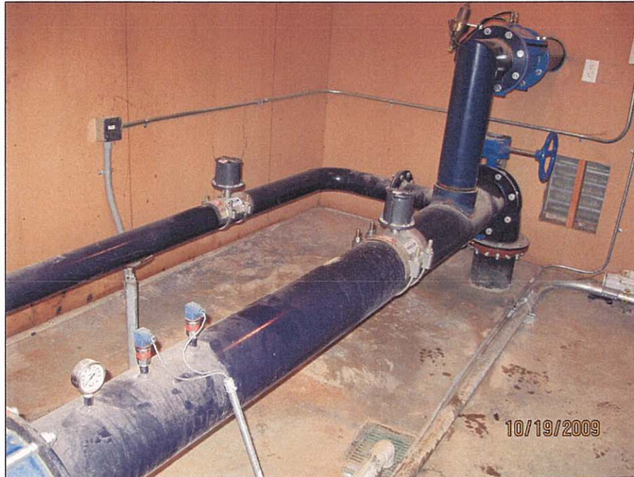
Big well discharge piping on right; small well discharge piping on left. Both pipelines equipped with McCrometer flowmeters. Flush line discharges to outside of pump house through pipe on upper right. Discharge pipe to distribution system through floor on center right.
