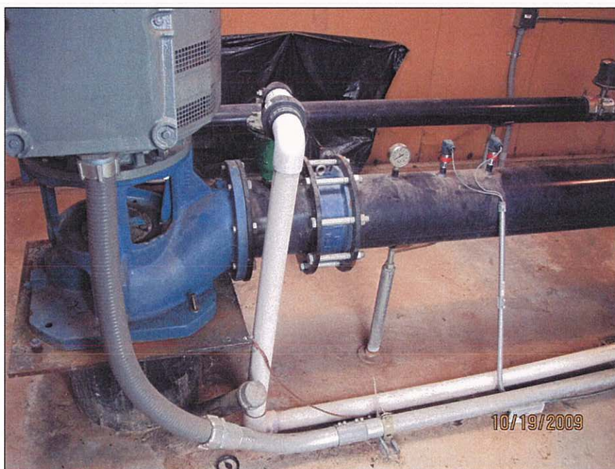
Big well and discharge piping.
