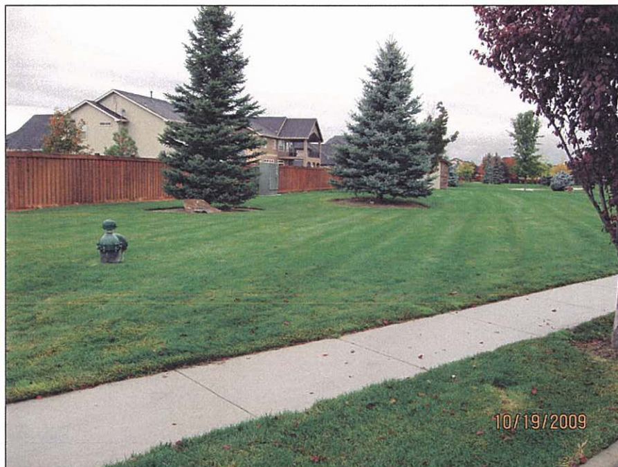
Small (8-inch) well on center left. Pump house in background on right.
