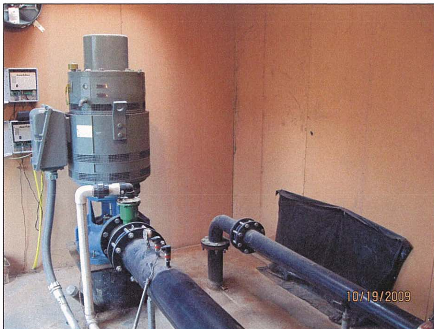
Big (16-inch) well on left equipped with 100-hp vertical turbine pump. Incoming pipeline from small (8-inch) well on right.
