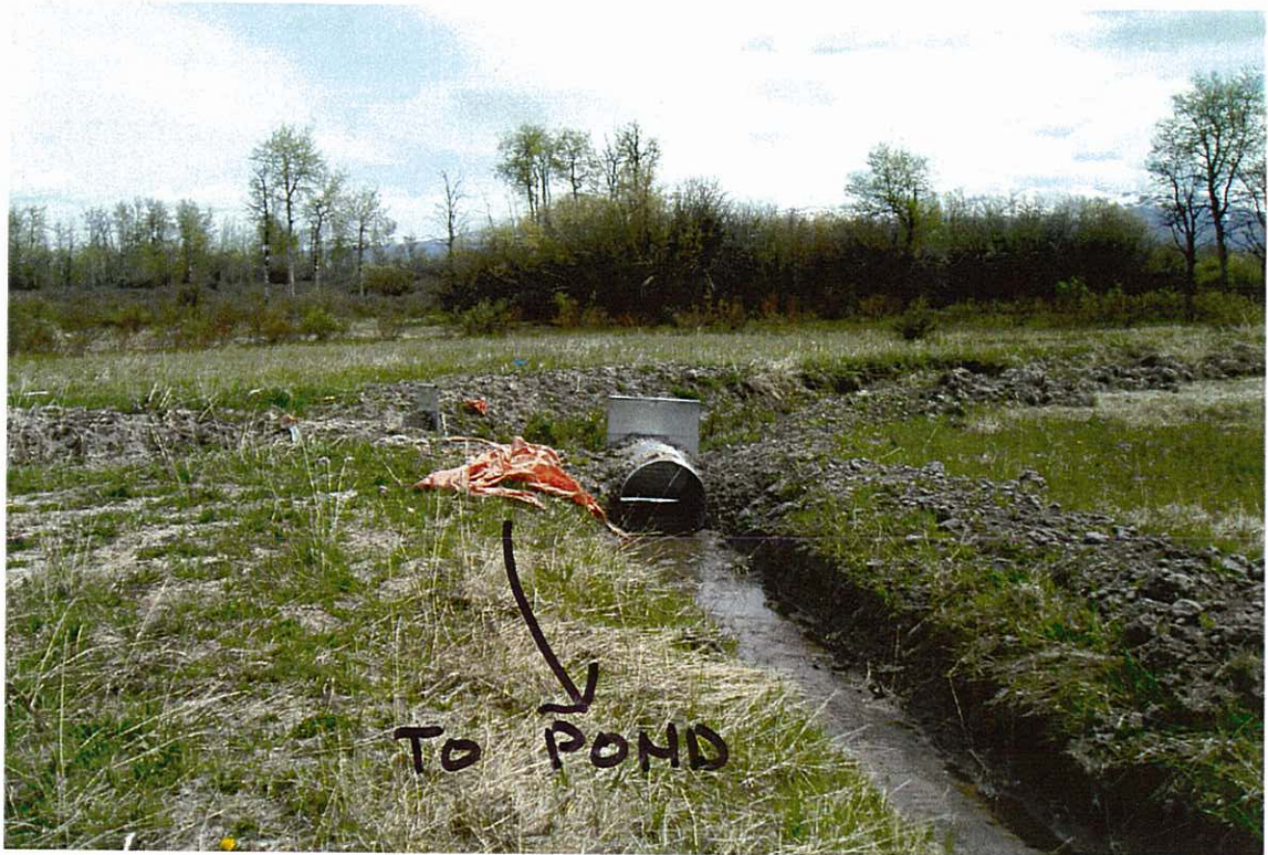
1. Headgate and ditch transporting irrigation water to Pond 2.
