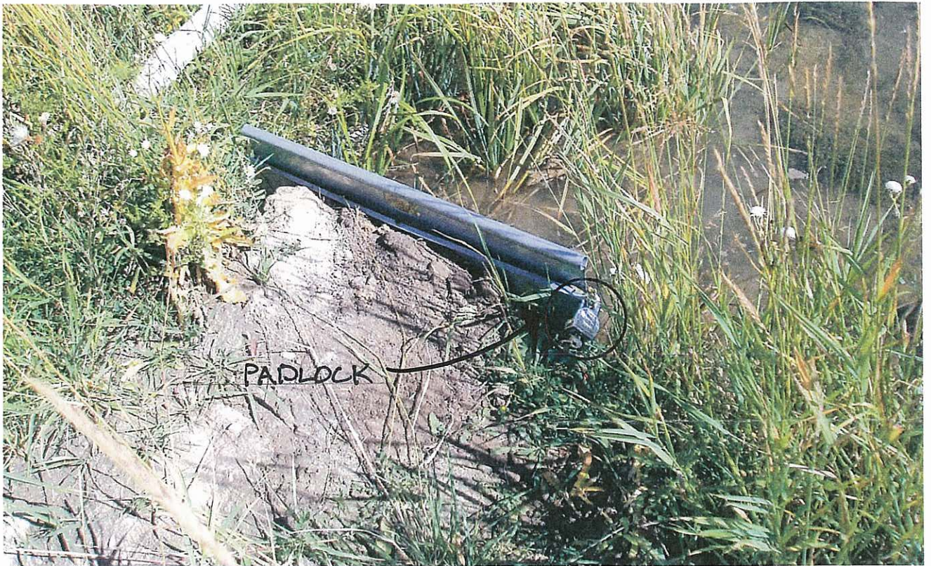
Headgate drilled so that a lock may be placed when gate is closed.
