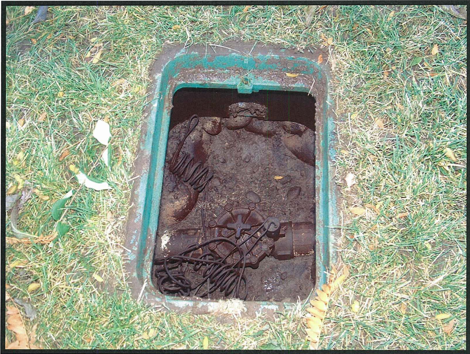
Sprinkler Valve Box
