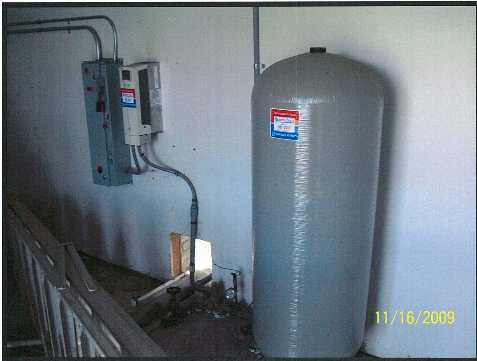
Pump Controlling Works and Pressure Tank
