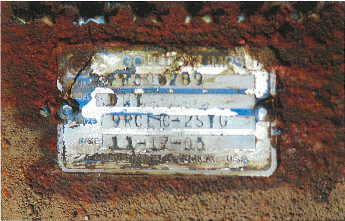
a) Town Ranch Supply Well #1 installed Goulds Pumps Model 9RCLC 2-stage pump nameplate.
