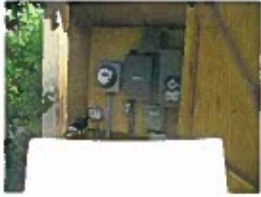
upper pump house.JPG
