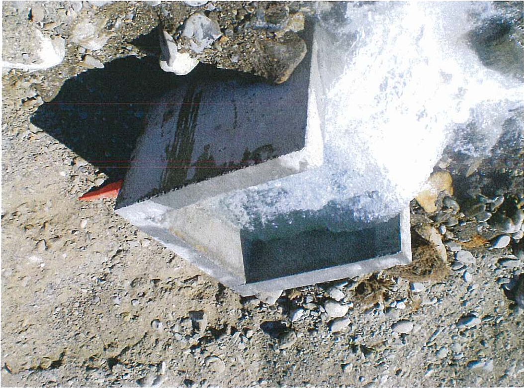
Discharge to pond / spa
