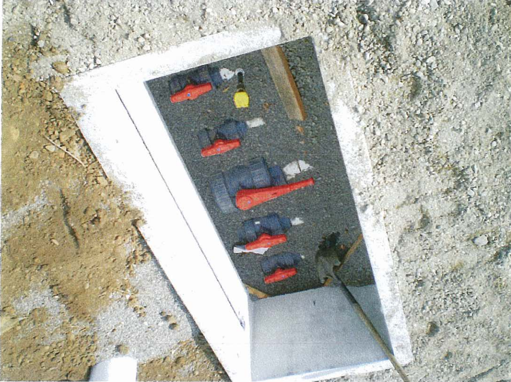
Main manifold. 4" valves to snowmelt system; 6" valve in mainline to pond.
