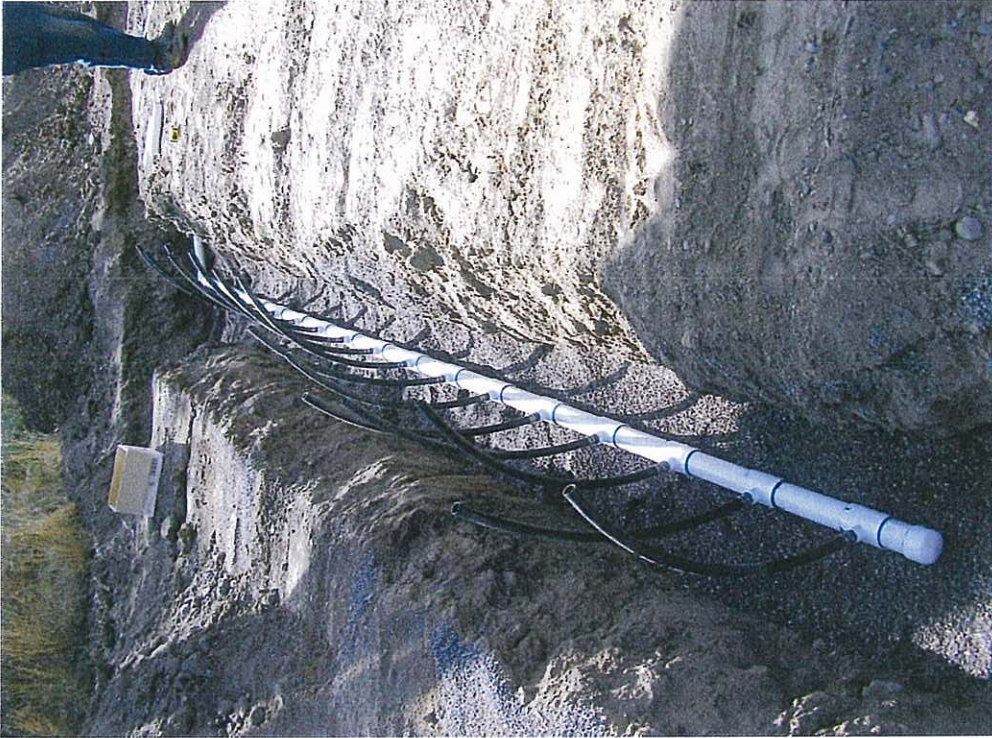
Example of snowmelt zone header (photo date 9/15/09)
