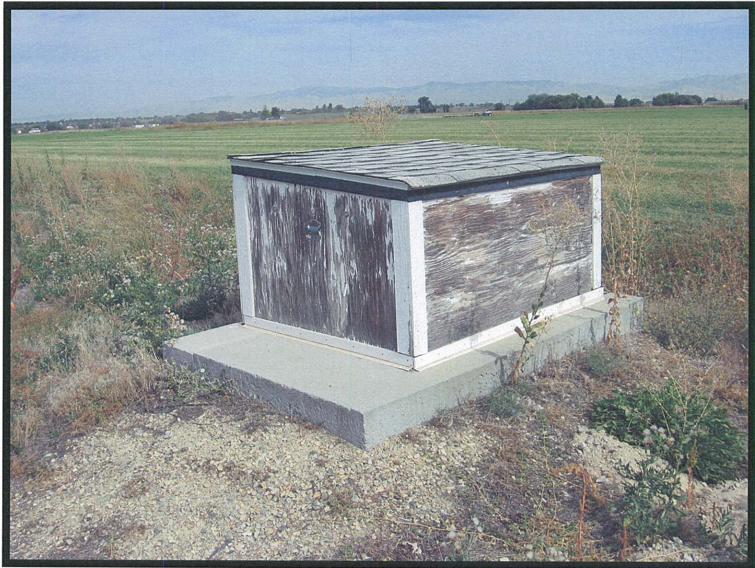
Well No. 2 (Back-up, Fire Protection Well)
