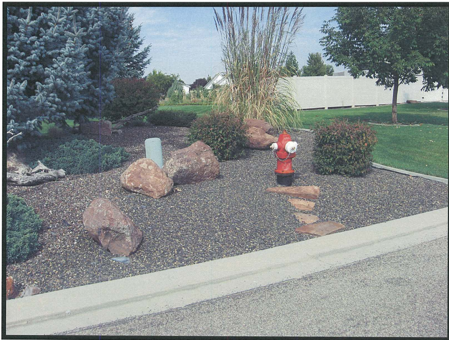
Fire Protection Hydrant & Stub for Lot 3, Block 1
