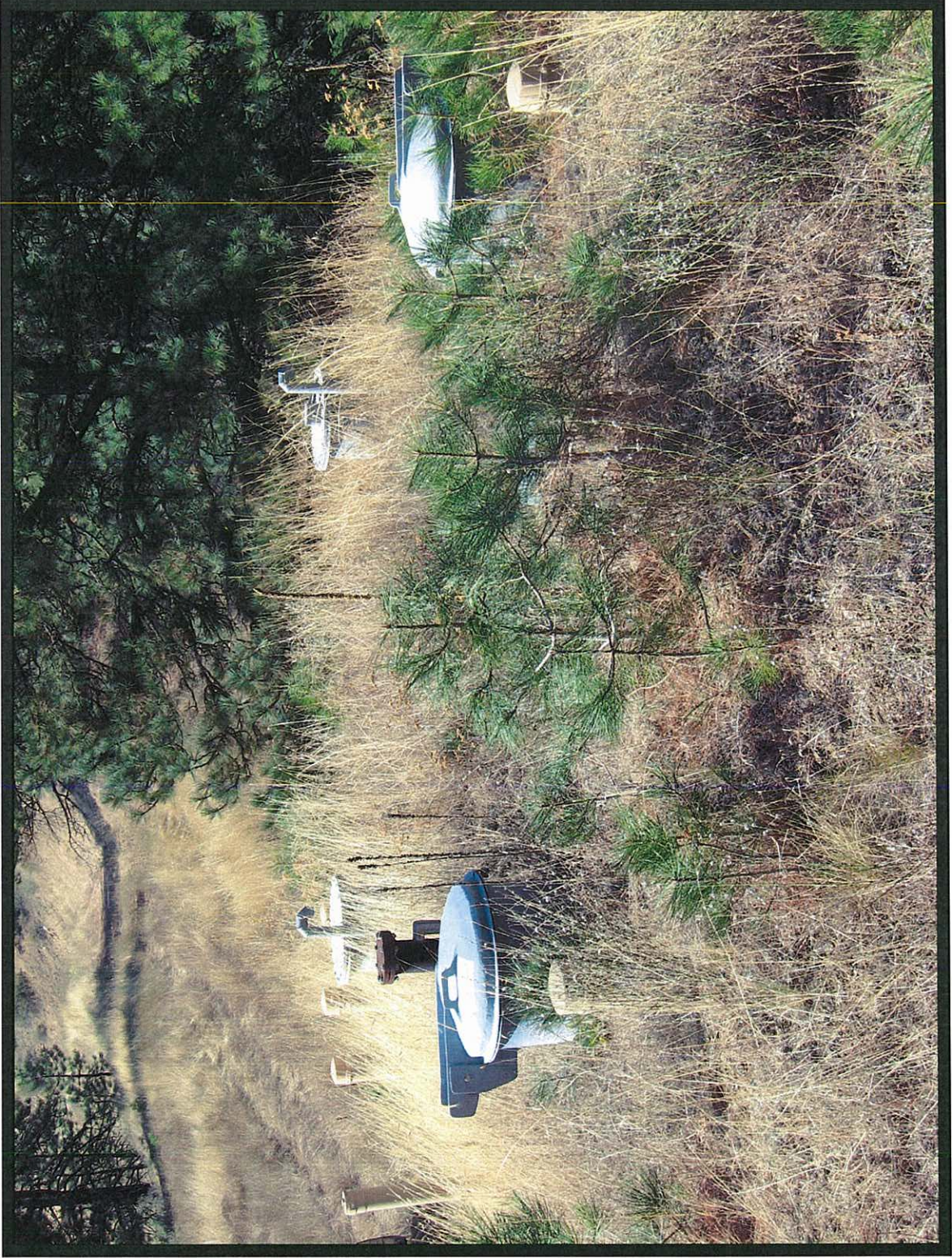
Lower Storage Tanks
