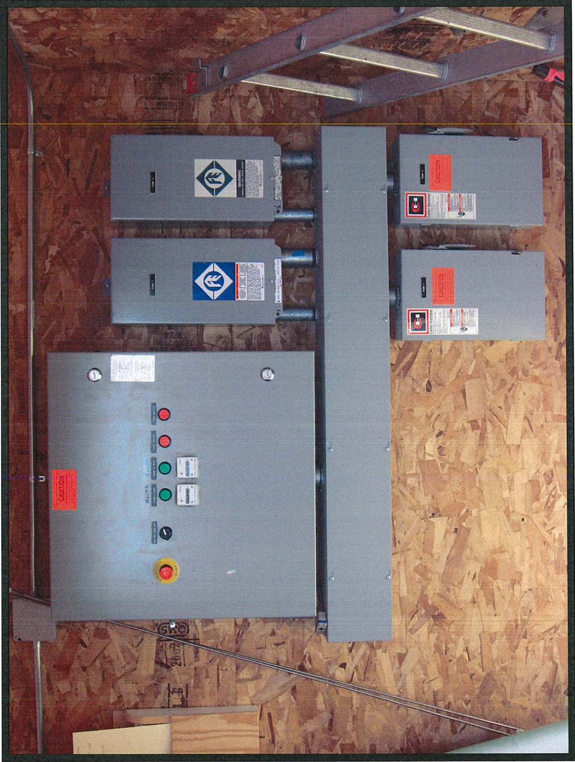
Controlling Works Inside Pump House
