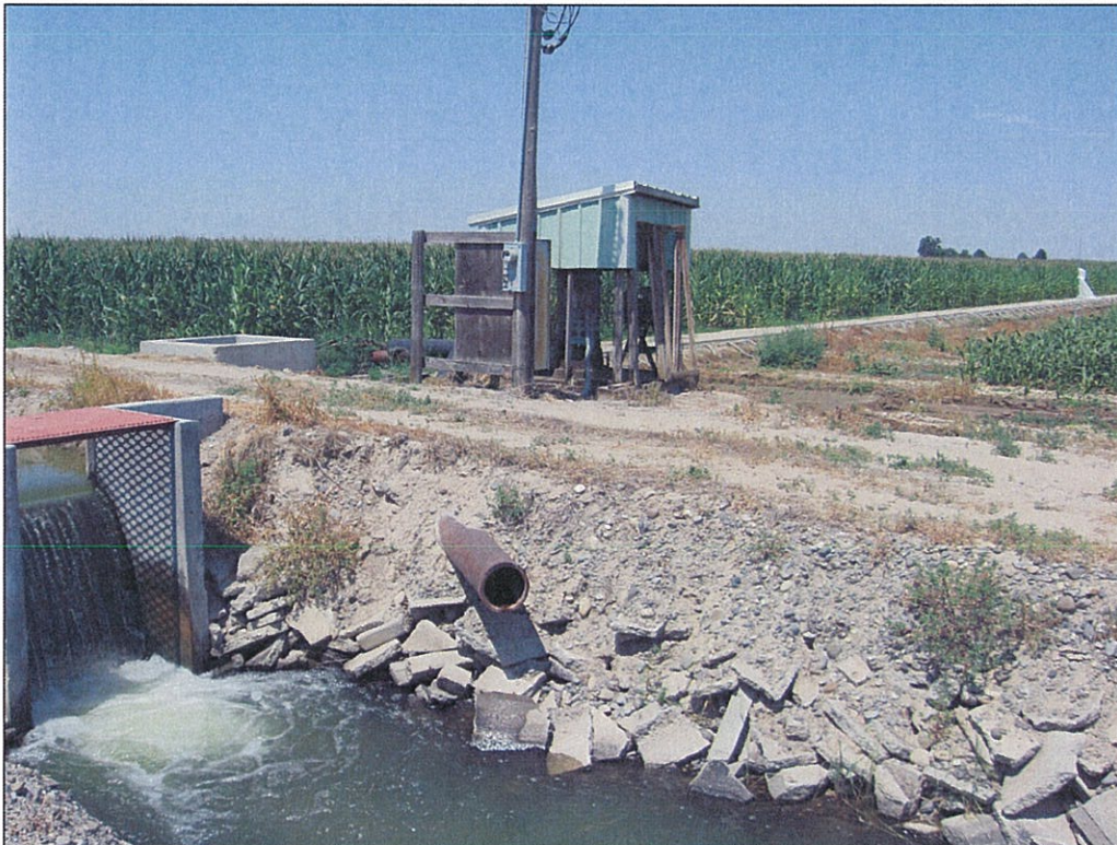
Figure 4: Well, facing northwest. Pipeline in foreground discharges to Paine Lateral, conveying water for use under this permit.
