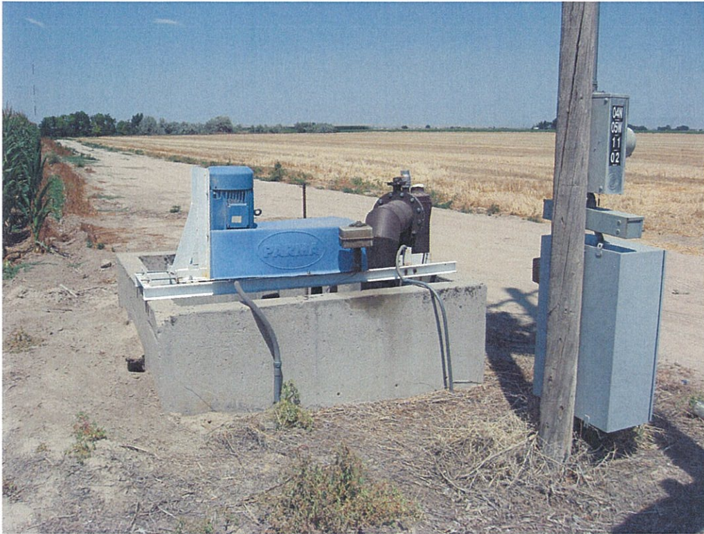
Figure 5: Parma Water Lifter re-lift pump. Photo taken facing northeast.
