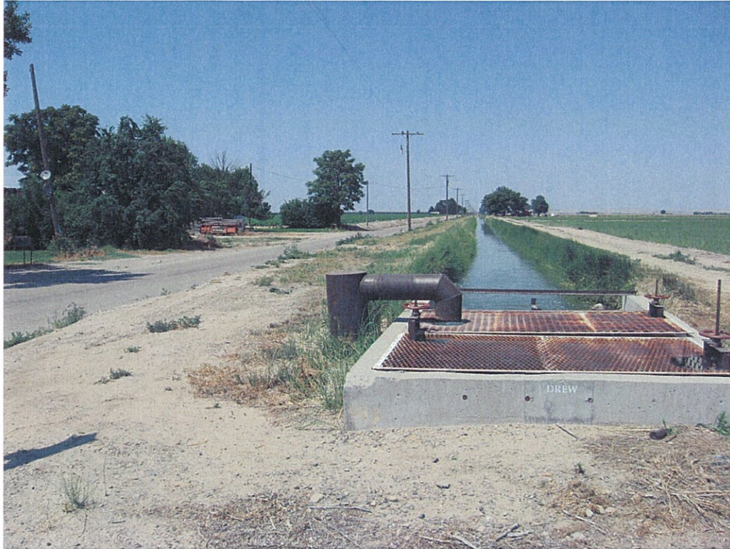
Figure 11: Photo of Drew Lateral facing north (downstream) taken at southwest corner of SWSW Section 12 (at intersection of Red Top Rd and Travis Rd). Black pipe discharging into box conveys water from the Parma Water Lifter in Figure 5 into the Drew Lateral.
