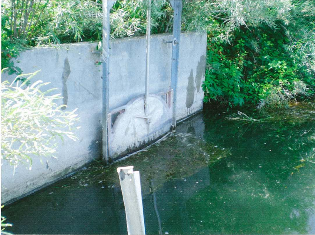
River side of diversion – 42" canal gate on concrete headwall
