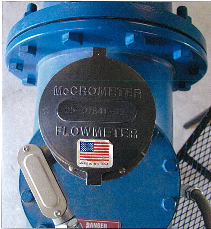
Figure 3. Photos of the 12-inch flow meter and line-pressure gauge for Meridian Supply Well #20-B
