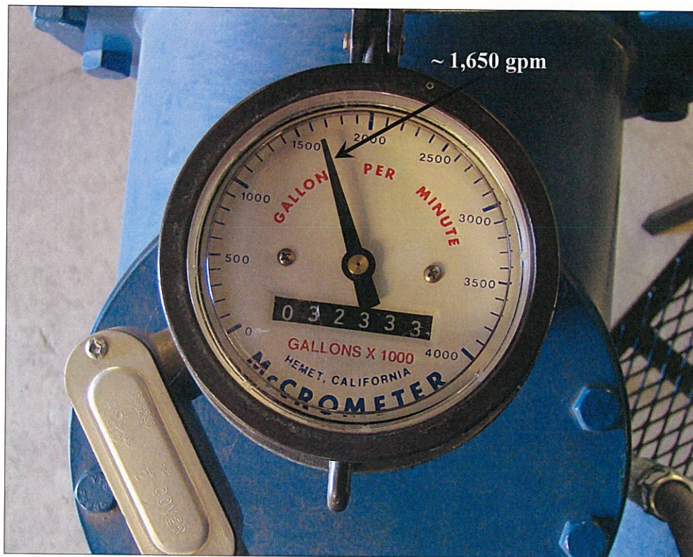
Figure 5. Photos of the Flow Rate and Pressure During Beneficial Use Exam of Meridian Well #20-B
