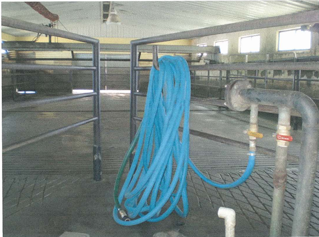
Holding pen. 1-1/2" hose used for flushing and clean-up.
