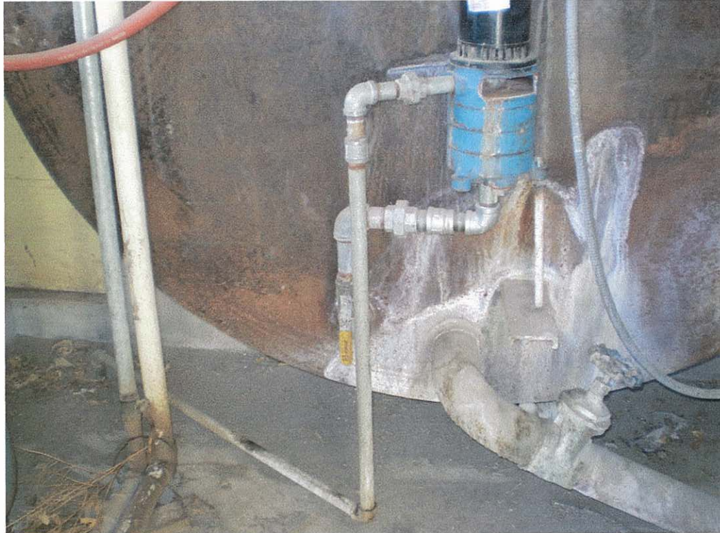
10,000 gallon tank and booster. 4" pipe on lower right leads to a second, larger booster pump.
