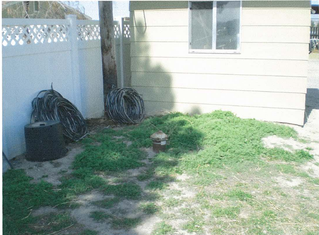
Well #1 and wellhouse
