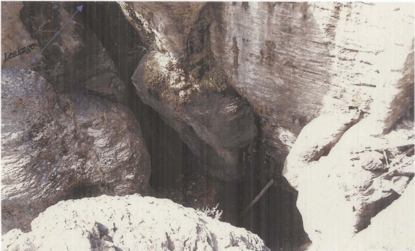
Photo #3: Leakage thru the right rock abutment, old outlet pipe at toe.
