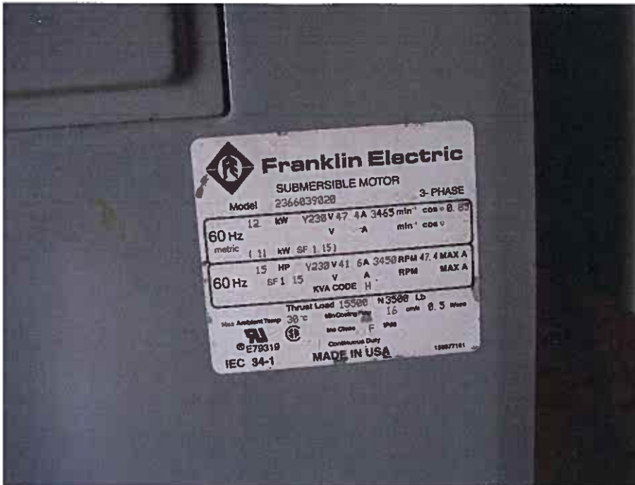
Specs on motor located in pump house.
