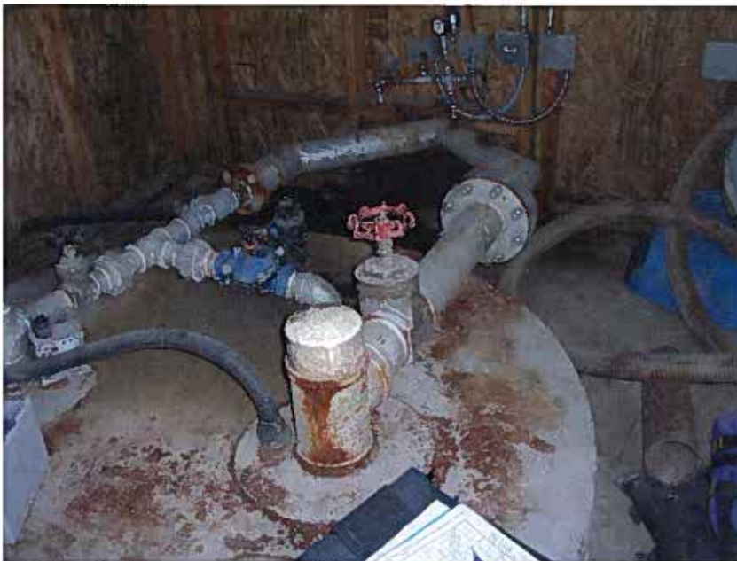
Pump and storage tank located in pump house on west side of pond.
