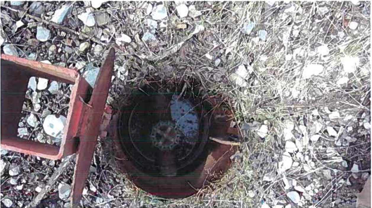
Photo 4 On/Off for system at POD
