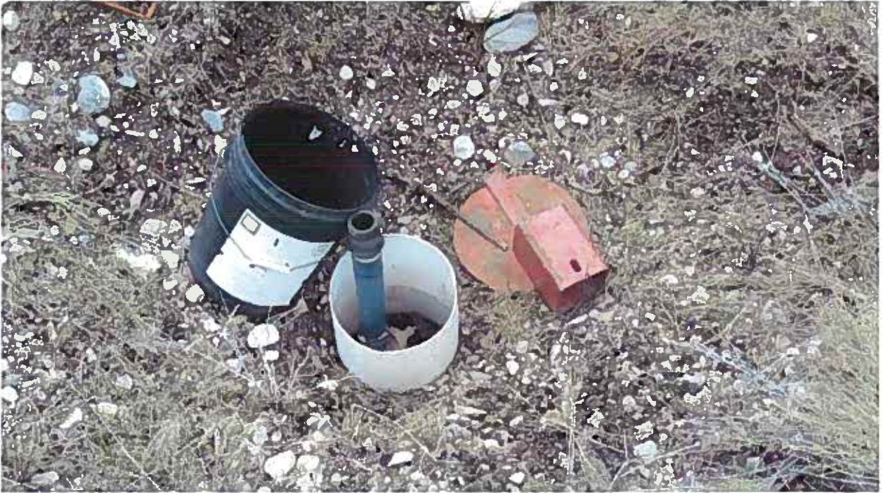
Photo 3 Overflow Pipe at POD
