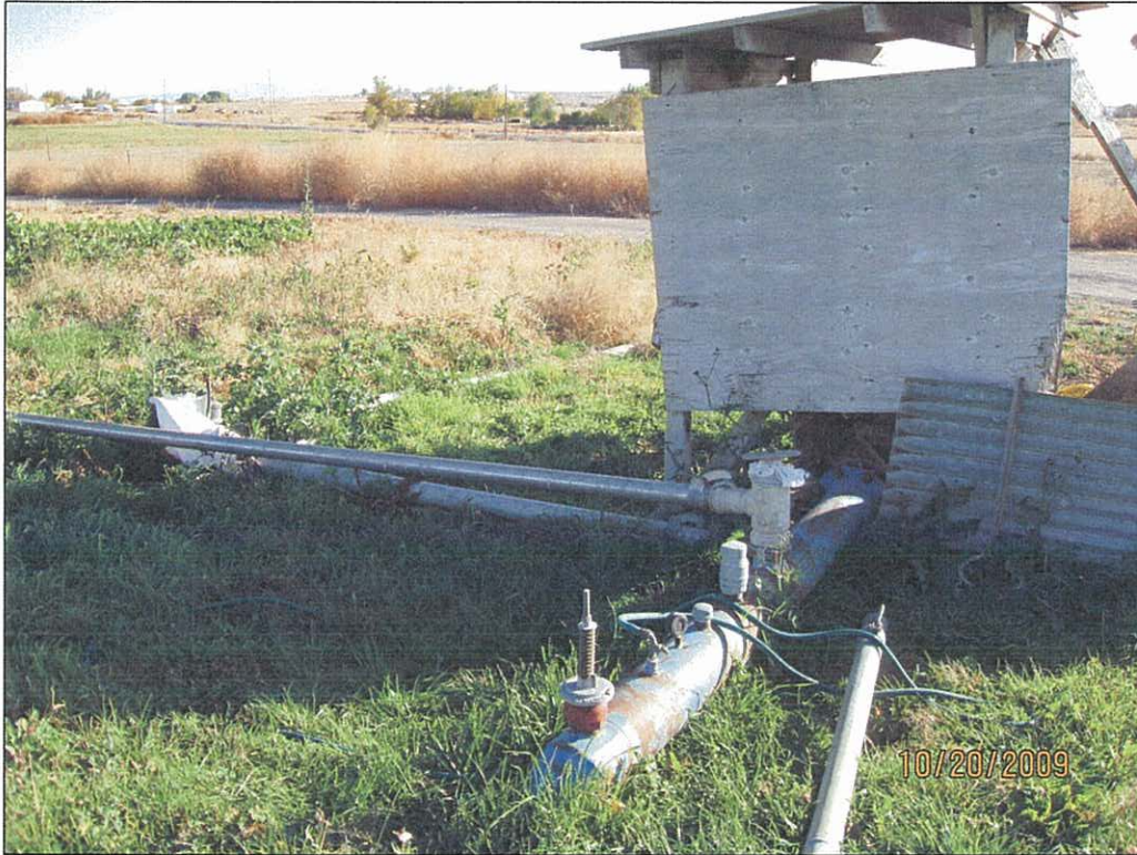
Photo 1: Well pump located in shelter. Diversion into Hat Butte Canal for this permit is accomplished by connecting the four-inch aluminum mainline lying on the ground to the riser valve.
